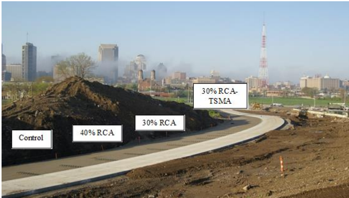
Figure 5-1. General view of the ramp approach with the reference section already in place
