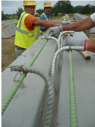
501 502 Figure 7. Photograph showing concrete rising through shear connectors and workers vibrating connectors to 503 consolidate SCC.
