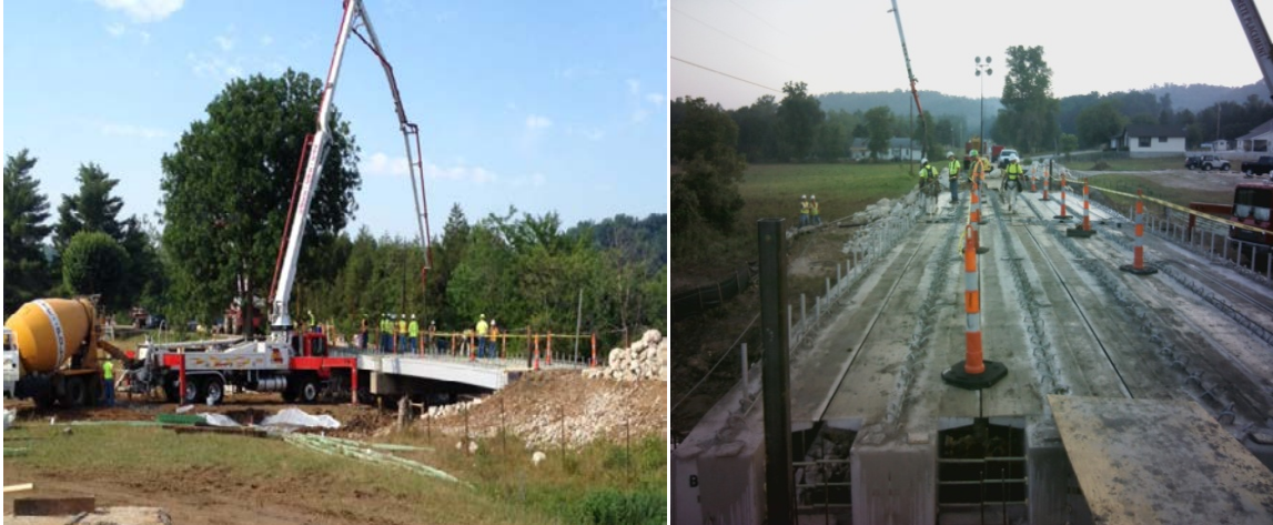
556 557 558 Figure 10. A & B: Photographs of concrete pump truck (left) and spans 1 &2 during concrete placement (right) for Bridge B0478
