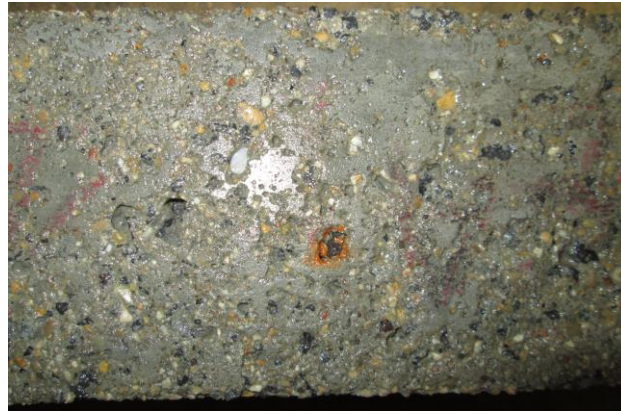
Evidence of corrosion in and EAF slag particle in Prism 1
