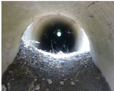
(f) Culvert is exposed due to a separated end section
