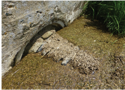
(d) End section of culvert completely submerged in water and debris
