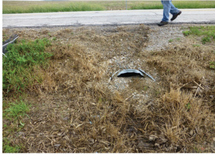
(a) Majority of end section filled with sediment reducing flow
