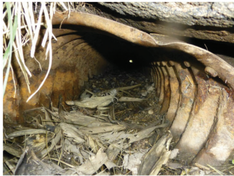
(e) Heavy corrosion causing potentially dangerous roadway conditions
