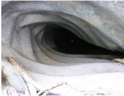
(c) End section of culvert pinched by farm equipment
