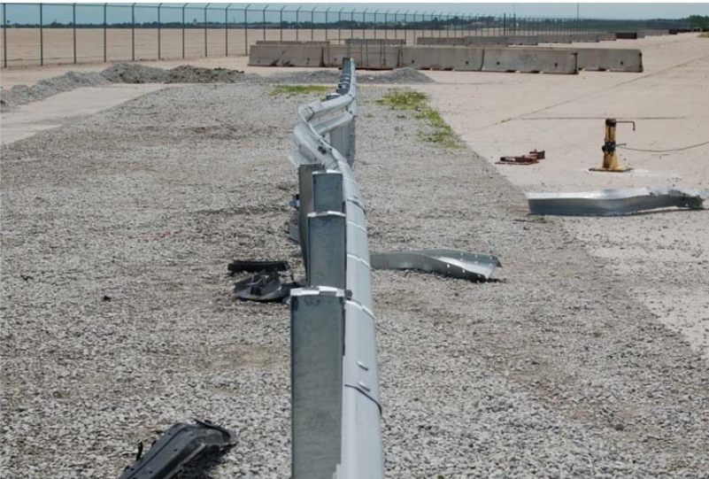
Figure 54. System Barrier Damage, Test No. MGSNB-2
