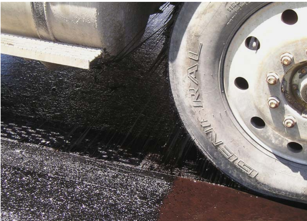
Figure 27. CQS-1HP Polymer Asphalt Emulsion as Applied in Section 1 & 2. Note the Strings of Tack Sticking to the Tire
