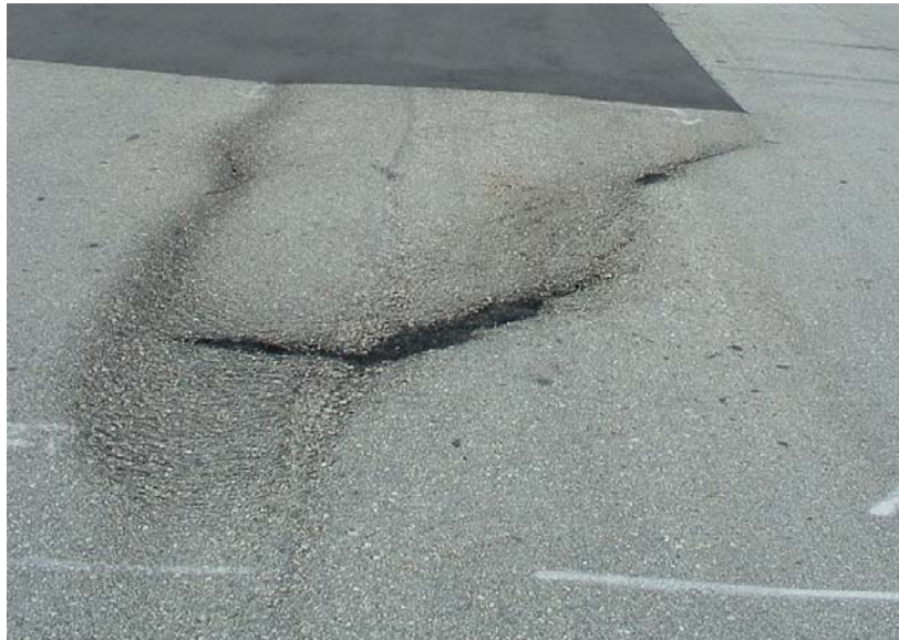
Figure 1. Slippage Failure Due to Poor Bond Between HMA Layers
