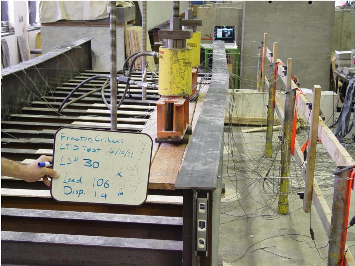
Figure 4-42. Deformed Bridge Under 106 kips of Load
