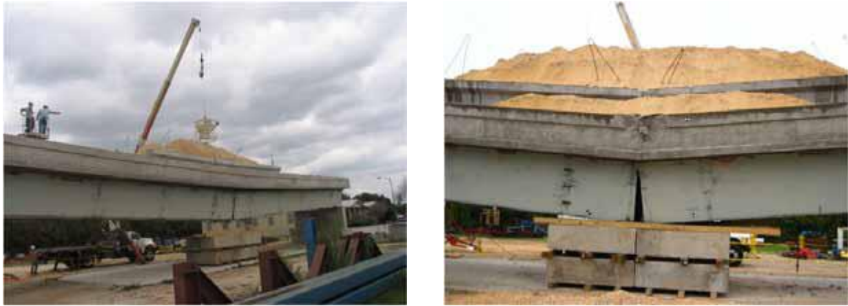
Figure 1-5. FSEL Third Bridge Fracture Test [Source: FHWA Report No.: FHWA/TX-10/9-5498-1]
