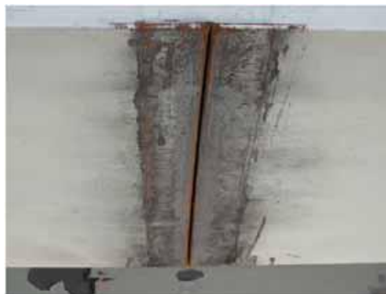
Figure 1-3. Bottom Flange Cut after the Explosion [Source: FHWA Report No.: FHWA/TX-10/9-5498-1]
