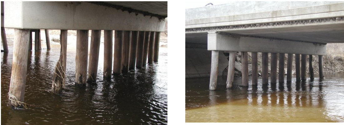
Figure 1.1: Examples of observed damages in Timber Piles in Nebraska
