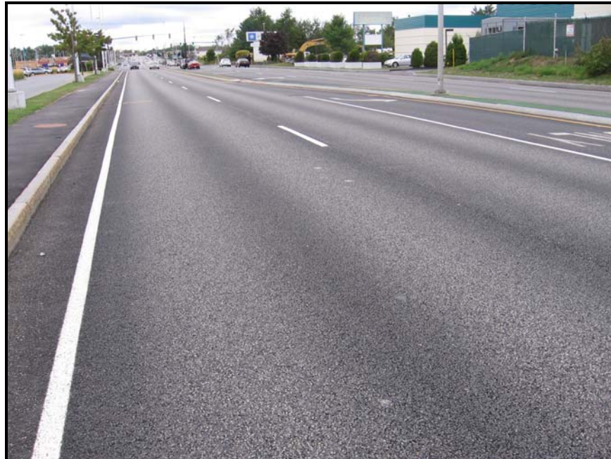
Figure 13 - OGFC Surface - Note wheel path discoloration.
