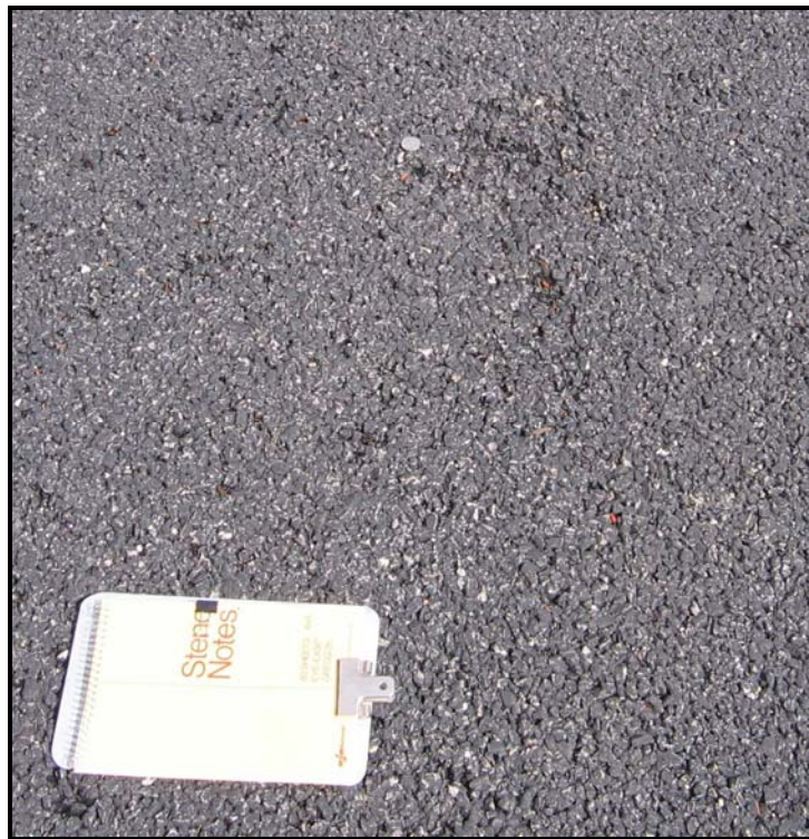
Figure 11 - OGFC Surface defects
