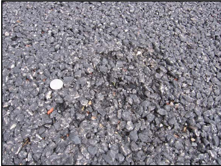
Figure 10 - Material loss in OGFC Surface
