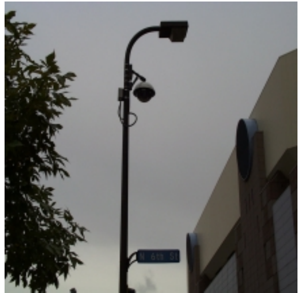
Surveillance Camera (Close-
