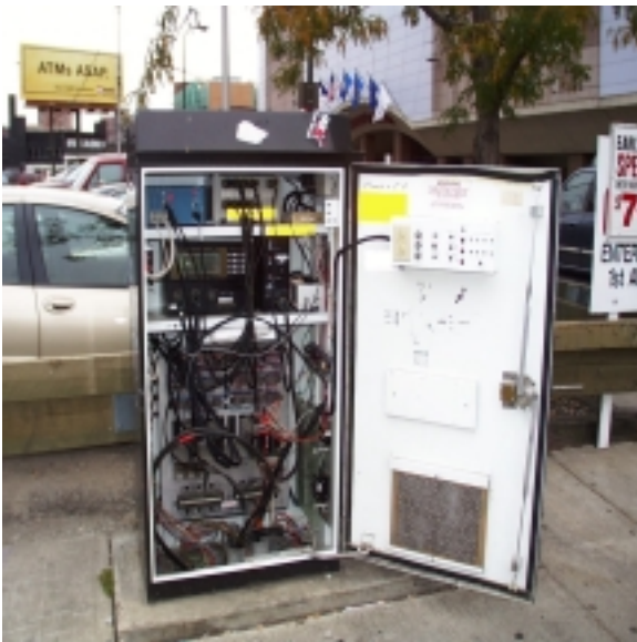
Intersection Controller Cabinet Equipment
