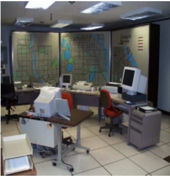
Minneapolis Traffic Control Center Computer
