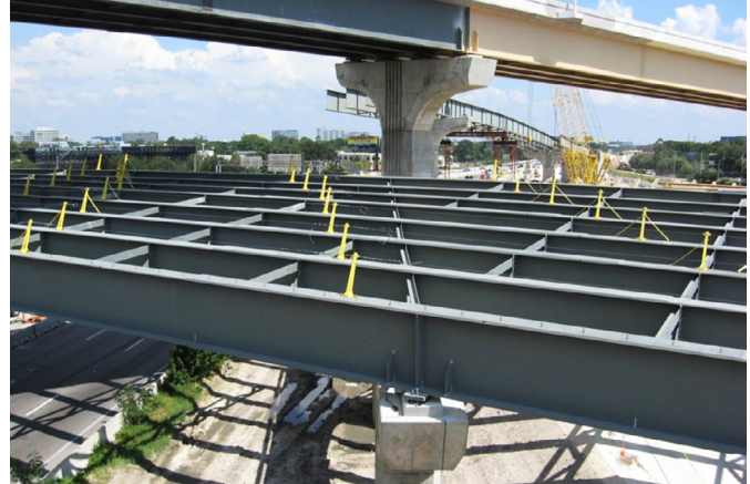
The cross-frames visible between this bridge's steel girders add stability while the deck is added.
