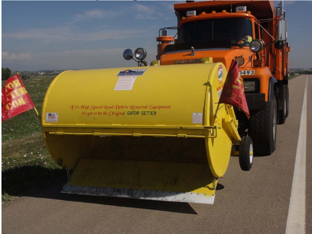
Figure 3: Gator Getter High-Speed Debris Removal Equipment
