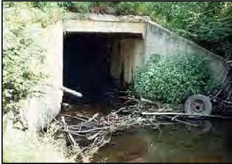
FIGURE 1.3 Box Culvert Obstructed with Driftwood
