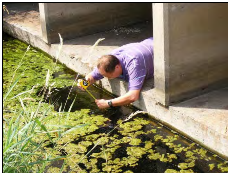
FIGURE 1.5 Scour Adjacent to Box Culvert
