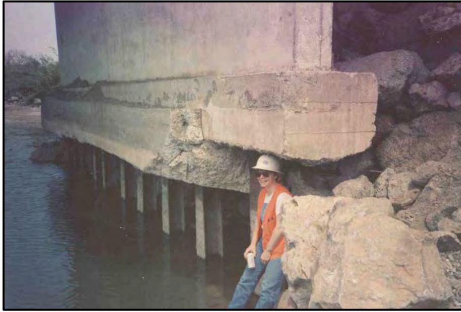
FIGURE 1.2 Scour Under Bridge Pile Bent
