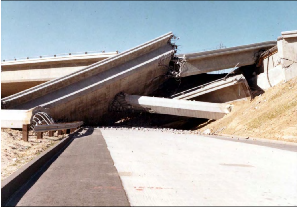
Figure 1.1: Example of 1971 San Fernando Earthquake Damage ( Courtesy of UCSD )
