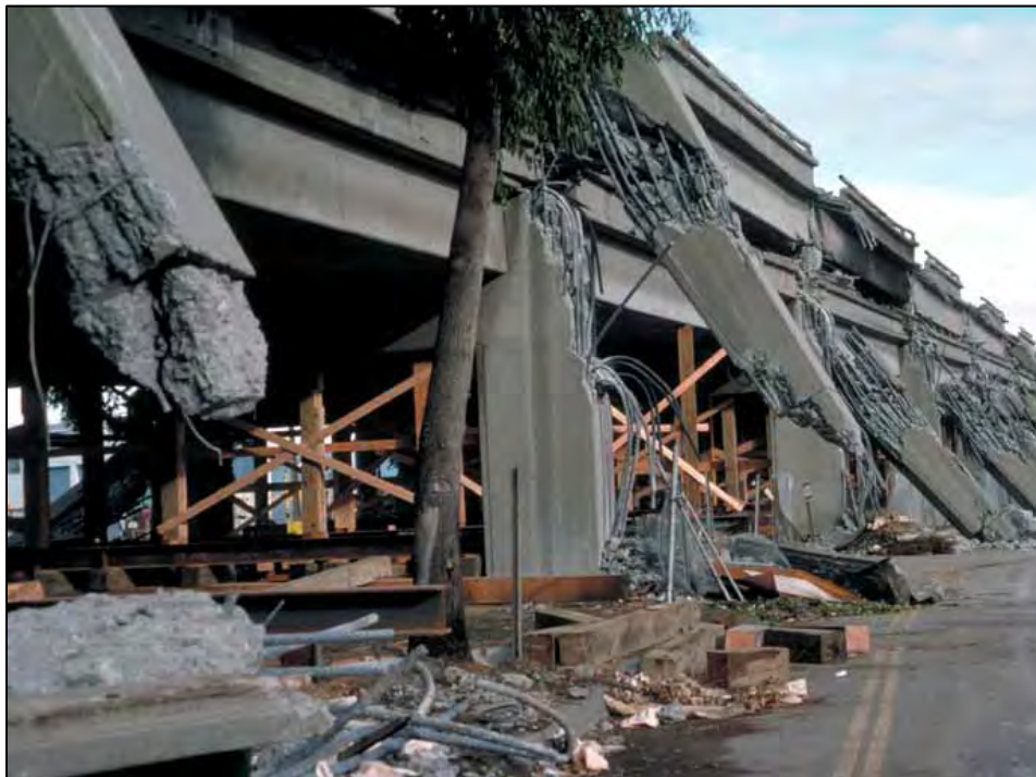
Figure 1.2: Example of 1989 Loma Prieta Earthquake Damage ( Courtesy of UCSD )
