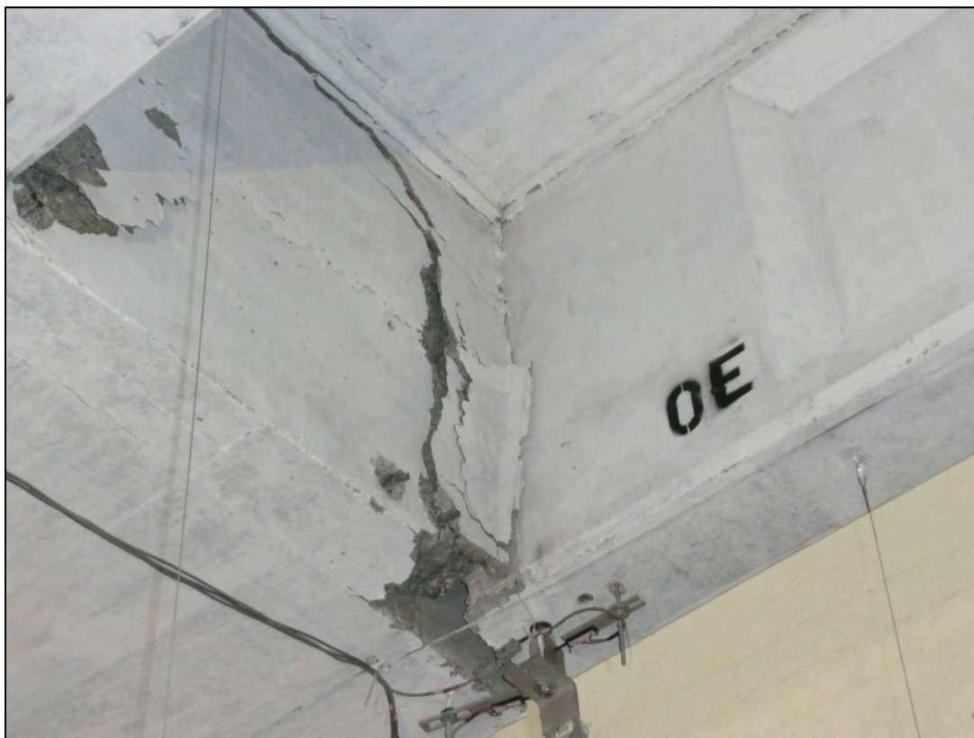
Figure 6.35: Damage to As-built Connection Exterior Girder at +2 in. Displacement
