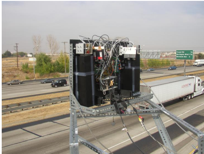
Figure 3-1: Detection System Mounted Above the Highway
