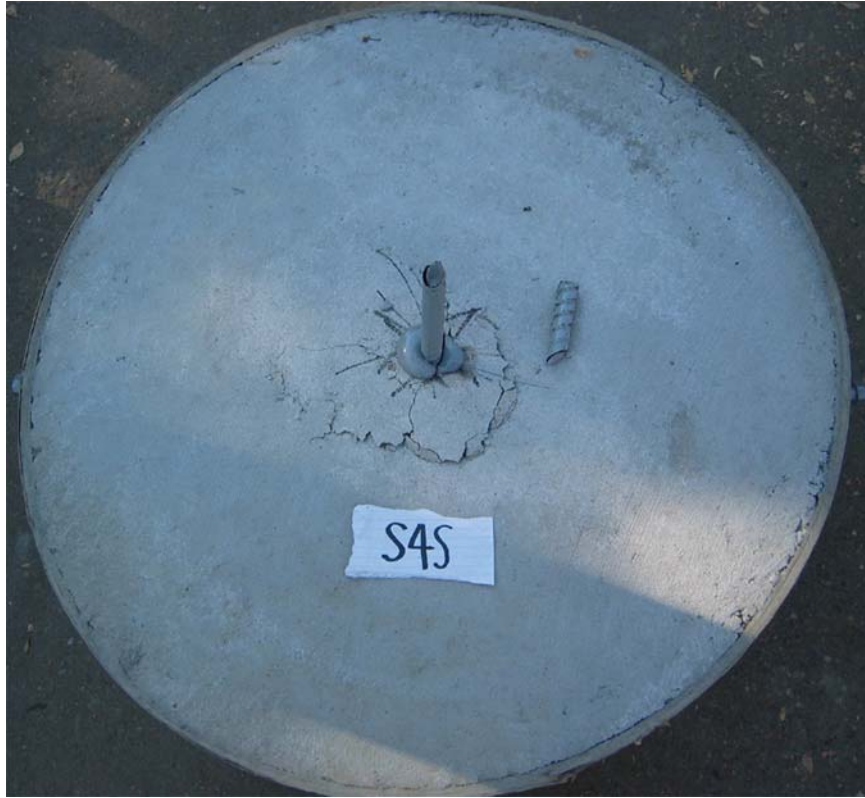
Figure A-5: Typical Rebar Failure
