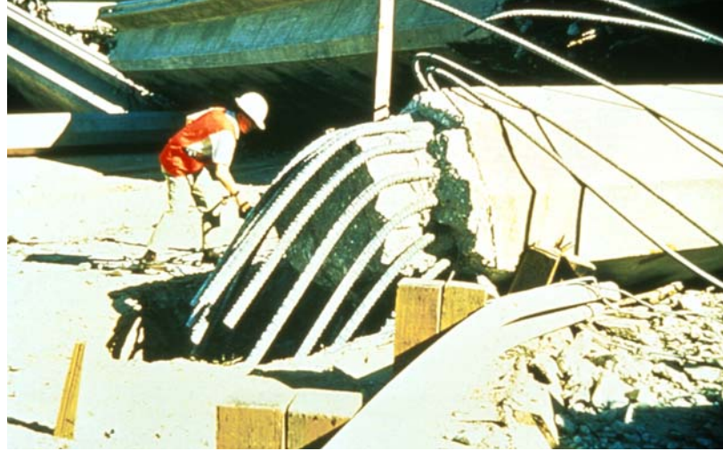
Figure 7-3. Pullout of column reinforcing steel.
