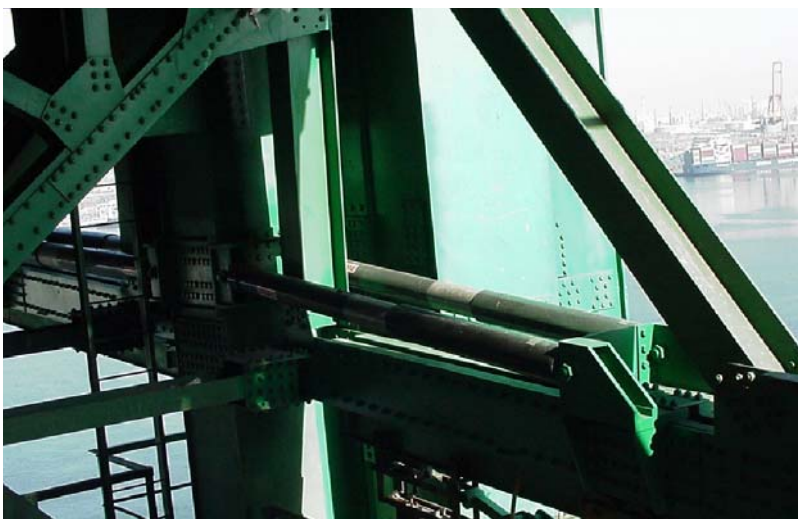
Figure 9-12. Viscous dampers installed at the Vincent Thomas Bridge in Los Angeles.
