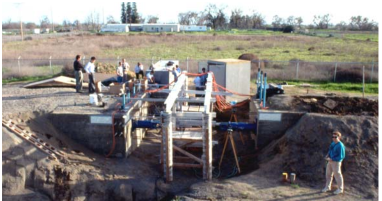
Figure 8-12. Large-scale field test to determine stiffness and capacity of end diaphragm abutments.
