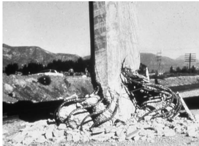
Figure 7-4. Single-column shear failure.
