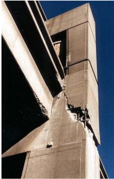
Figure 9-9. Joint failures, I-880 Cypress Street Viaduct, Oakland, in the 1989 Loma Prieta earthquake.
