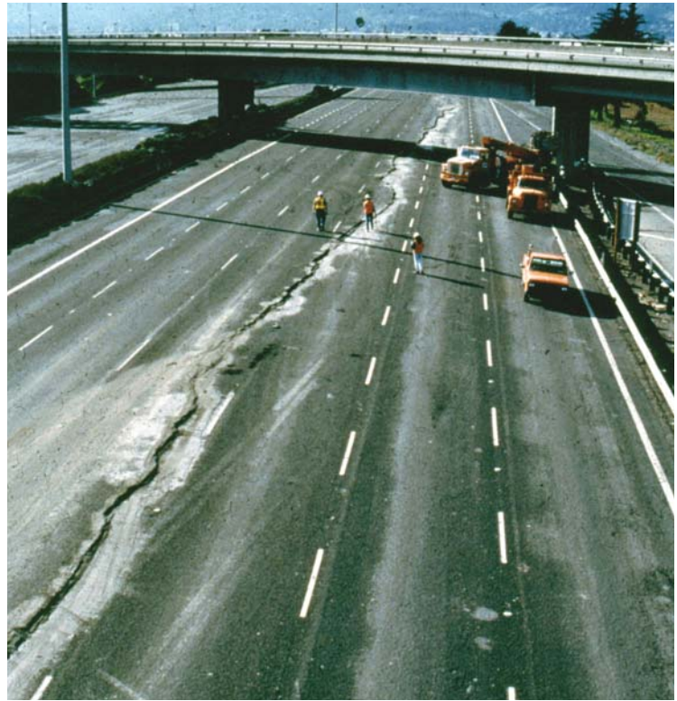
Figure 5-7. Liquefaction leading to lateral movement and cracking of pavement at the approach to the San Francisco-Oakland Bay Bridge during the 1989 Loma Prieta earthquake.
