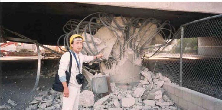
Figure 9-8. Shear failures of short columns in the 1994 Northridge earthquake.
