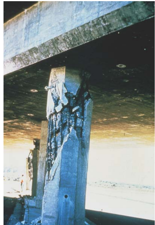
Figure 7-5. Multiple column shear failure.
