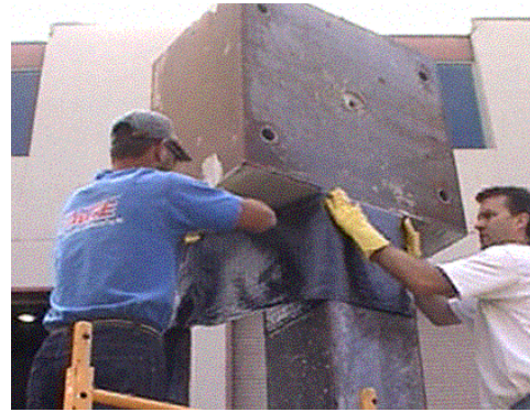
Figure 9-17. Seismic retrofit of a masonry building using wet lay-up of fiber reinforced polymer (FRP) jackets for column retrofit.
