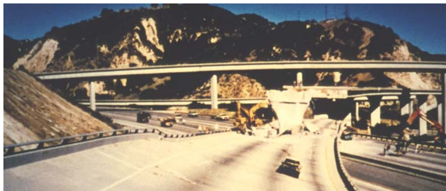
Figure 7-18. Collapsed end spans over Interstate 5 in the 1994 Northridge earthquake.
