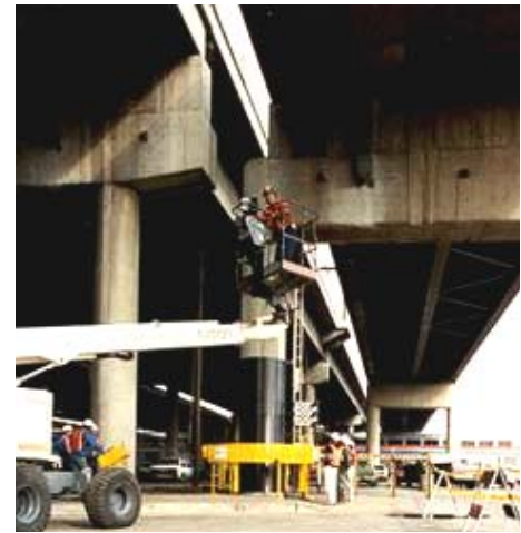
Figure 8-2. Carbon fiber jacketing of two-column bridge bent on the I-10, Santa Monica Viaduct.
