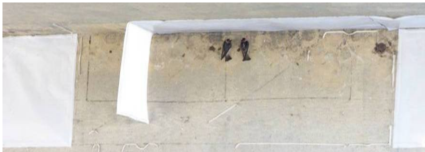
Figure 15. PTFE sheets detaching from the highway structure surfaces and cliff swallows building nests.
