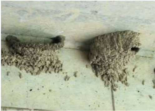
Figure 1. Partial and completed cliff swallow nests on underside of highway structure.
