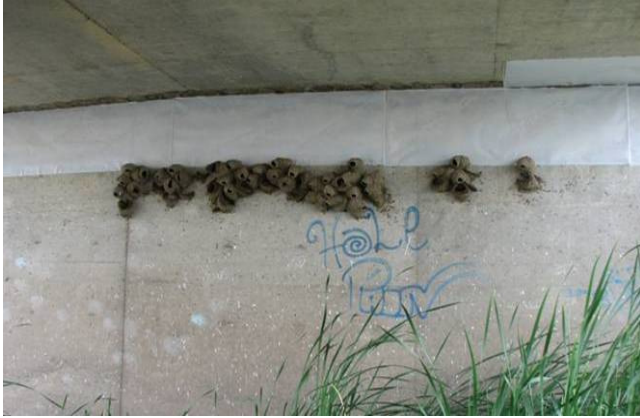
Figure 16. Completed nests below the bottom edge of PTFE treatments on a pier wall.
