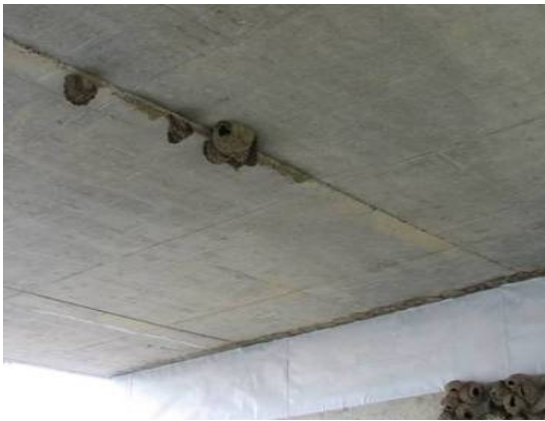
Figure 17. Completed nests on an overhead concrete seam at a PTFE-treated site.
