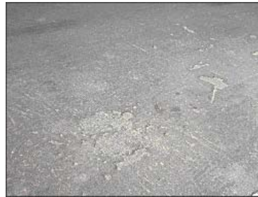
b) Delamination from a False Slurry
