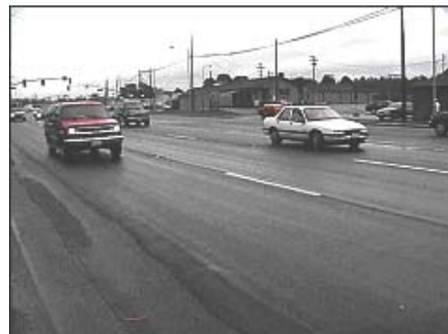
b) Poor Quality Edges and Shoulder
