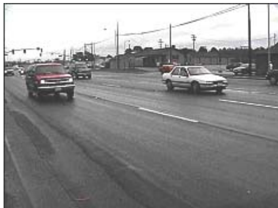
b) Poor Quality Edges and Shoulder
