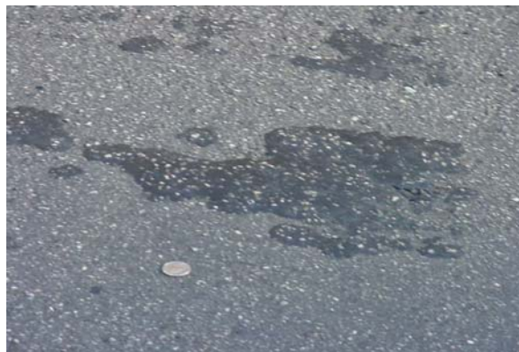
Figure 1-28 Bleeding/fat spot (seal coats)
