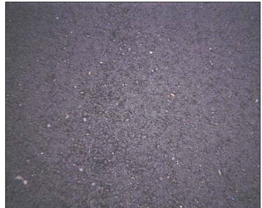
New tight DGAC surface. Application rates of more than 0.06 gal/sq yd could result in slick surface. Not suitable for fog or rejuvenator seal on high speed facilities.
