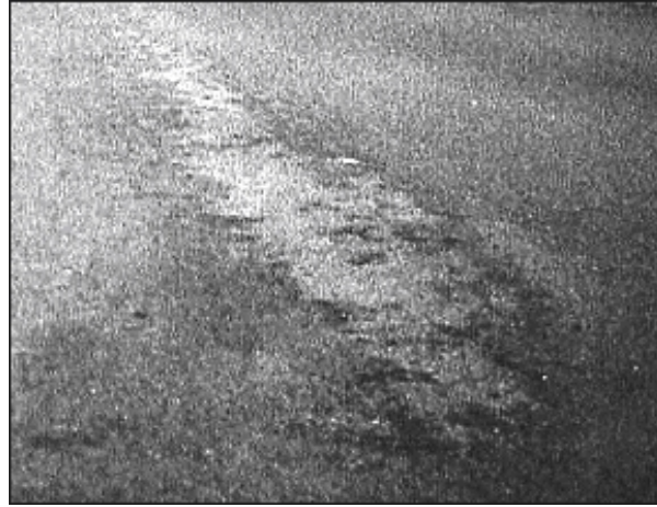
Figure 8-17 Traffic Damage Caused by Early Trafficking
