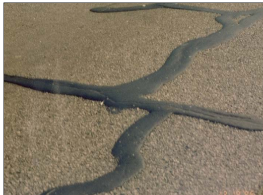
Figure 4-23 Poor Workmanship – Raised, Bumpy Sealing
