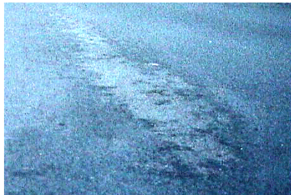
Figure 1-29 Delamination (seal coats)
