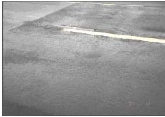
b) Low Quality Transverse Joint
