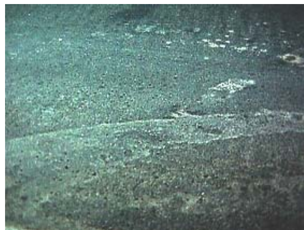
Figure 8-18 Damage Due to Post Application Heavy Rain with Shear
