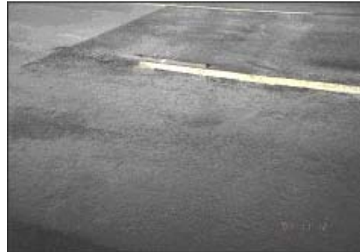
b) Low Quality Transverse Joint
