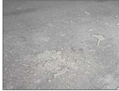
b) Delamination from a False Slurry
