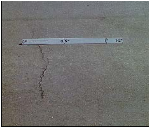
(Direction of Travel →) Figure 4-3 Transverse Cracking
