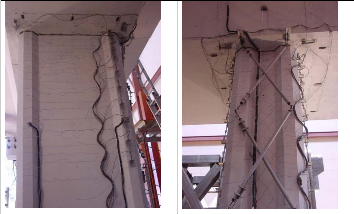
Figure 6.2 Marked crack pattern on north and west faces of column at \mu=2
