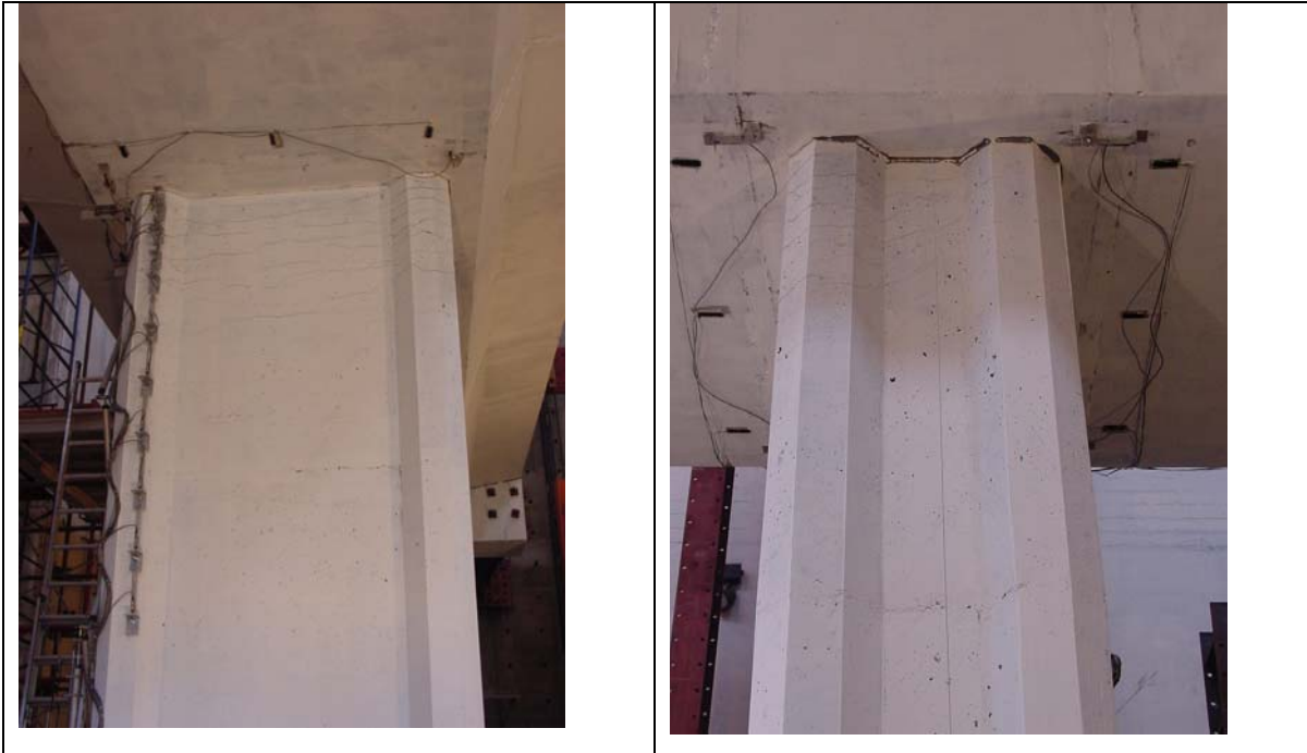
Figure 6.4 Unmarked crack pattern on south and east faces of column at \mu=4
