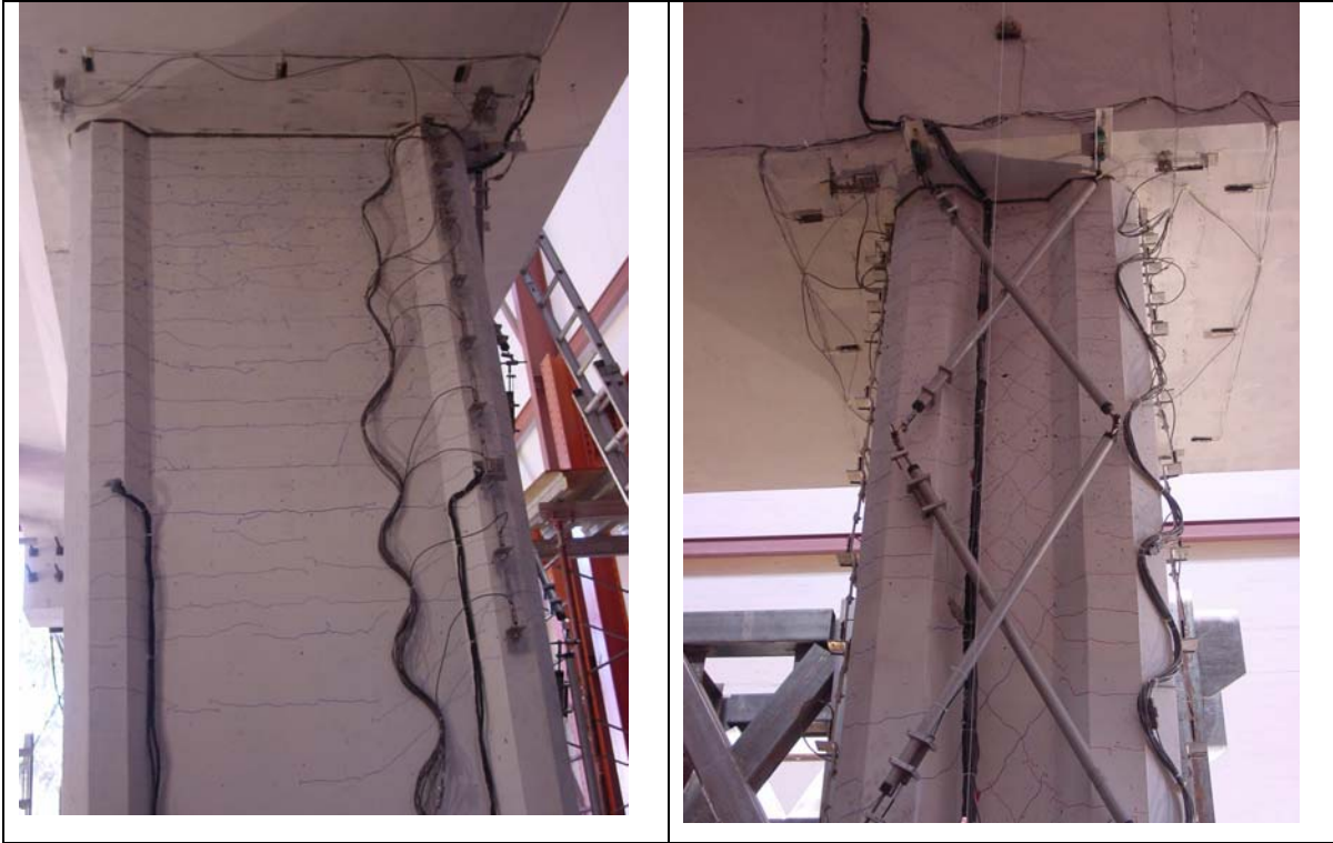
Figure 6.3 Marked crack pattern on north and west faces of column at \mu=4
