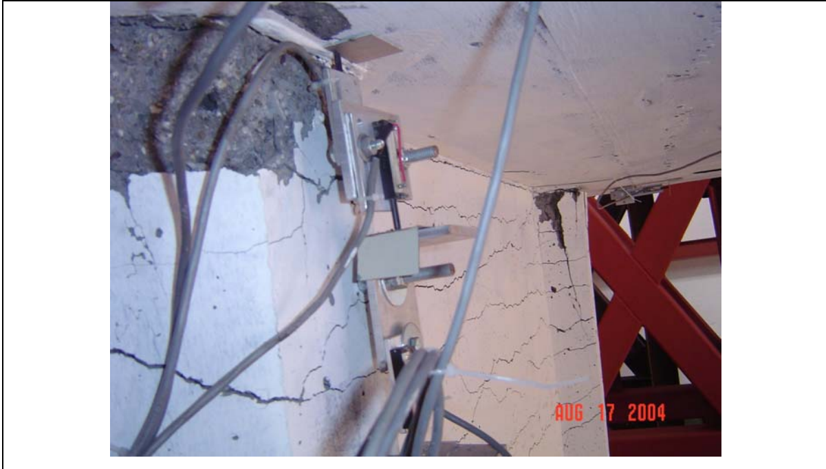
Figure 6.6 Spalling of column south face corner regions at \mu=5
