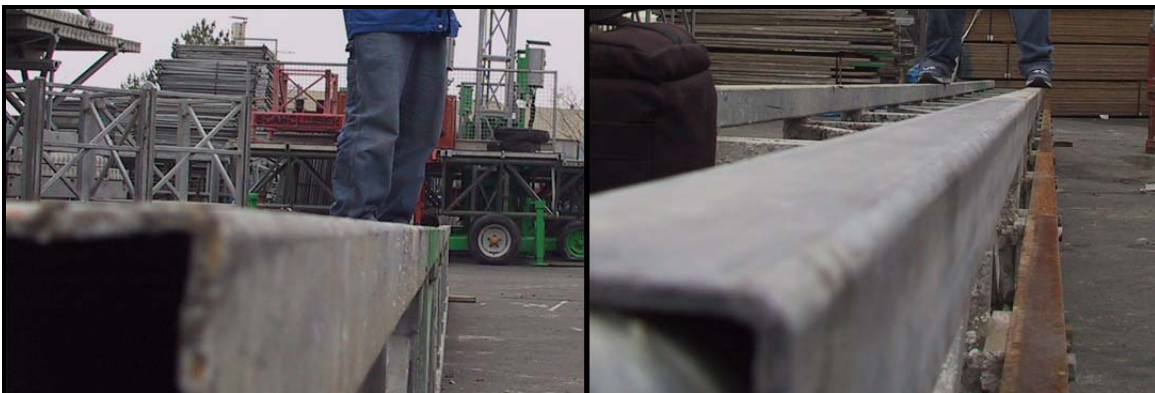
FIGURE 10-A8, DEFLECTION FROM LOAD AT CENTER OF SCAFFOLDING SPAN
