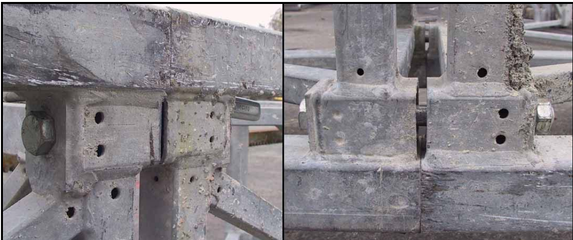
FIGURE 13-A8, TWO SCAFFOLDING PIECES BOLTED TOGETHER
