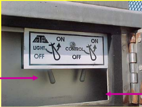
Police\Light Switch Panel
