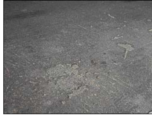
b) Delamination from a False Slurry
