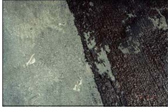
b) Dirty surfaces Result in Poor Adhesion (Delamination)
