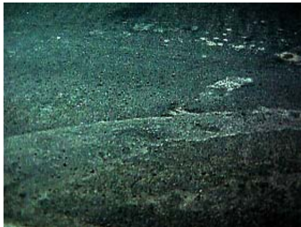
Figure 24: Damage Due to Post Application Heavy Rain with Shear
