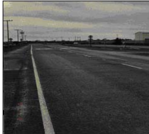
b) Poor Quality Longitudinal Joints
