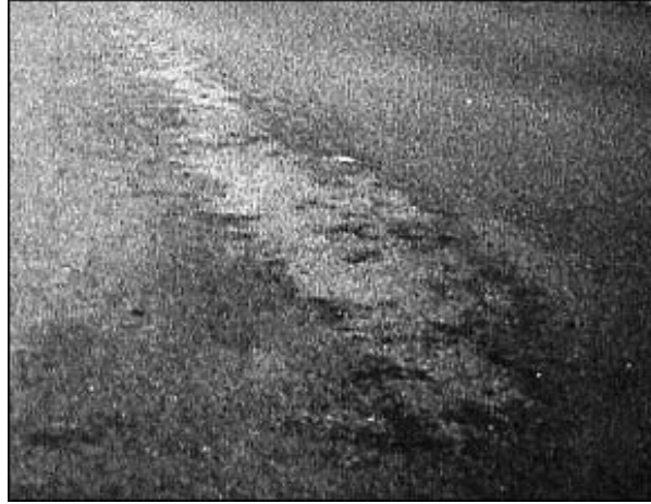
Figure 23: Traffic Damage Caused by Early Trafficking
