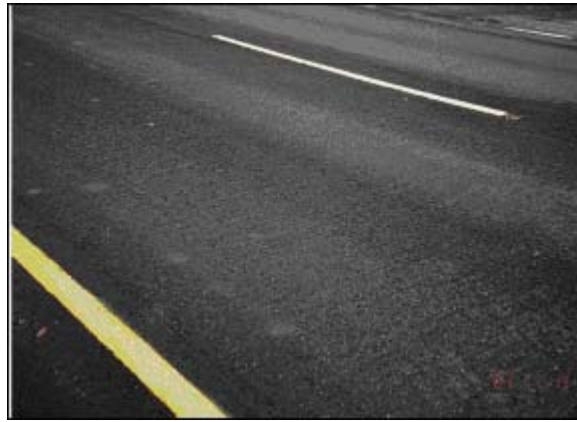
Figure 22: Wash Boarding Effect
