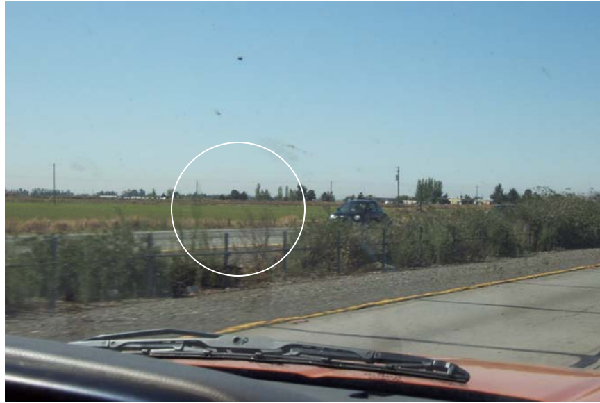
Figure 1.4 Undesirable Vegetation Around and Under Guardrail
