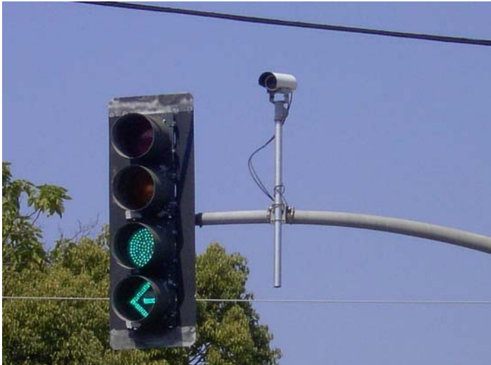
Figure 2. Components of Iteris Vantage (monochrome camera) installation at California and Foothill test site: East-facing video camera, video processors in Type 334C cabinet, overall intersection view.
