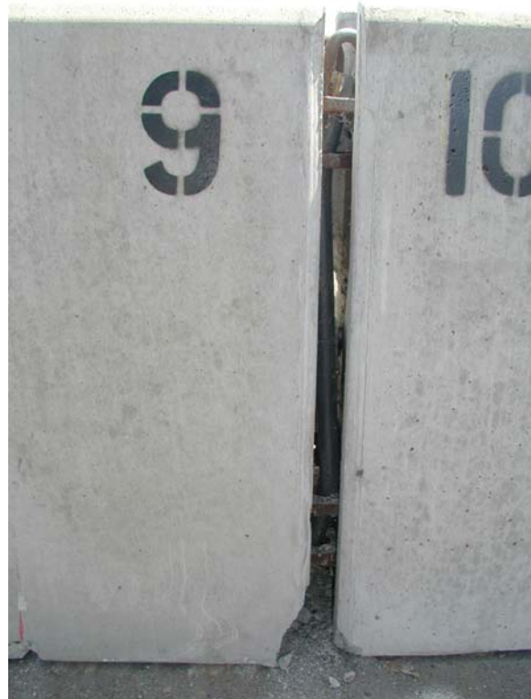
Figure 2-15 – Backside of Joint 8-9 showing Minor Concrete Spalling and Bent Pin (mislabeled)
