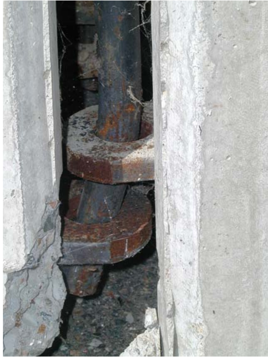
Figure 2-16 – Close-up of Bent Pin at Joint 8-9
