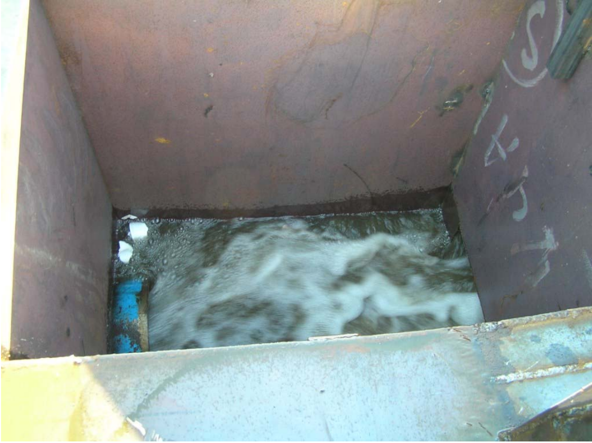
Fig. 6.44: Gross solids being carried over the splash plate and deposited in outflow tank.
