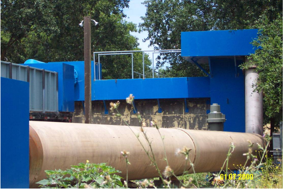
Fig. 2.5: Square pipe supply to first receiving tank.
