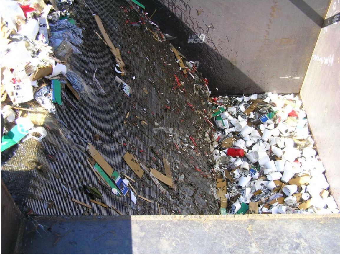
Fig. 6.41: Screen clogging with Q=1.1 cfs and 90% loading.
