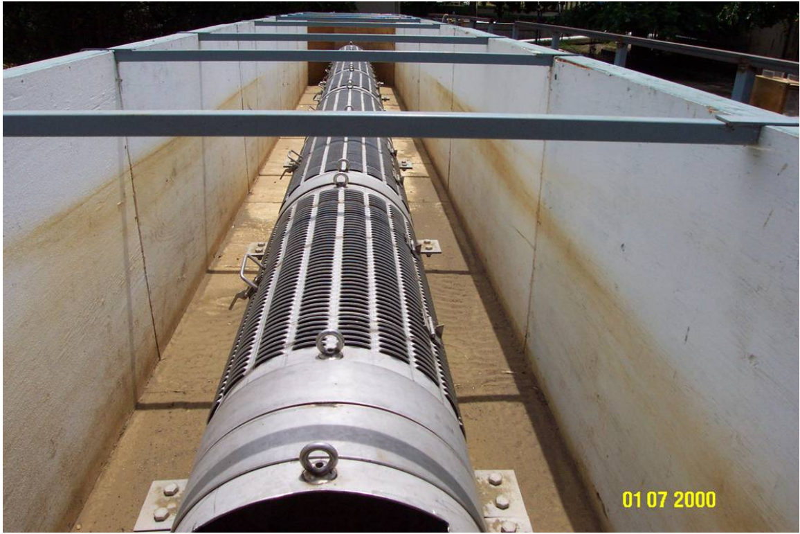
Fig. 2.10: Inside of vault showing Linear Radial device.
