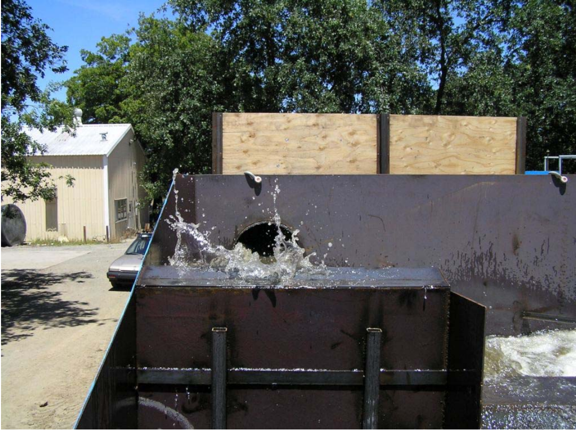
Fig. 6.33: Overflow over splash plate for Q=9.0 cfs.
