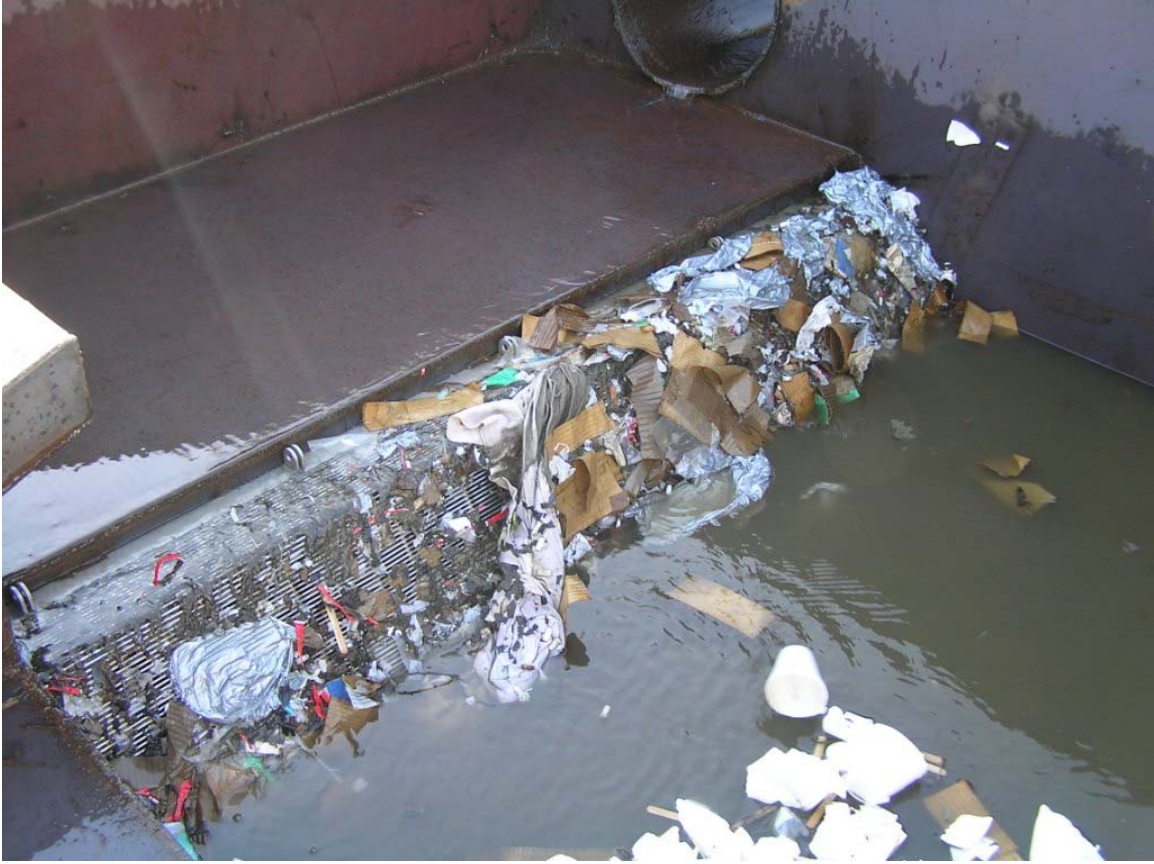
Fig. 6.48: Aftermath of Q=5.5 cfs and 50% loading.
