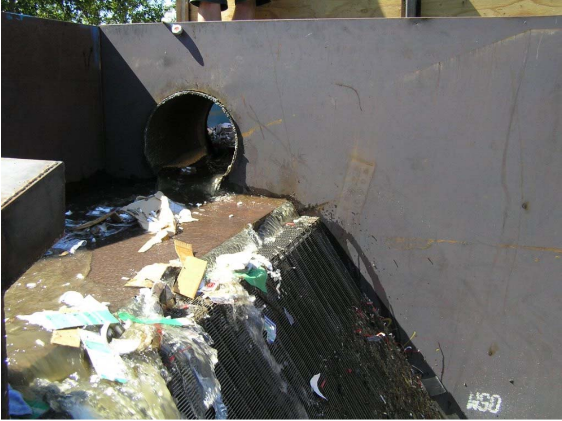
Fig. 6.35: Gross solids not being cleared entirely at low flow rates ( Q=1.1 cfs, 10% loading).
