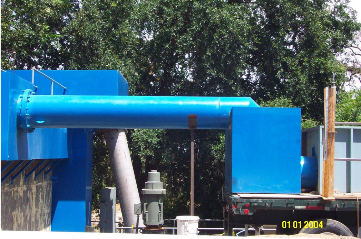
Fig. 2.8: Delivery to trash insertion tank
