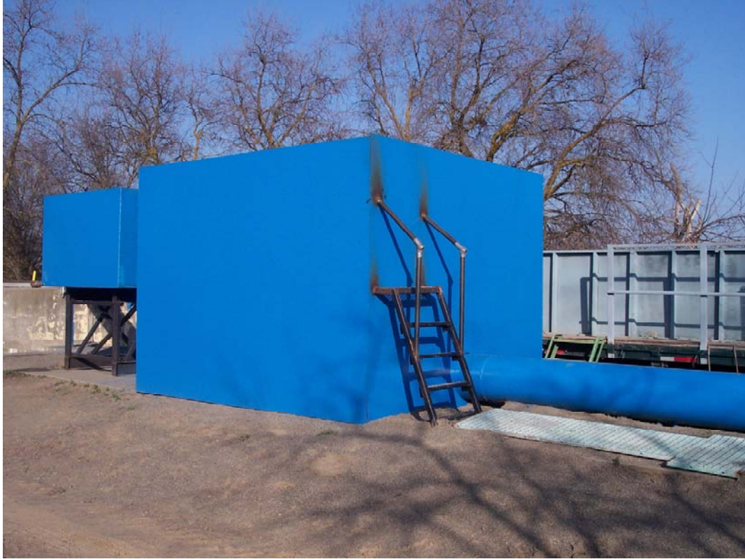
Fig. 2.16: Vault containing Type 1 inclined screen.
