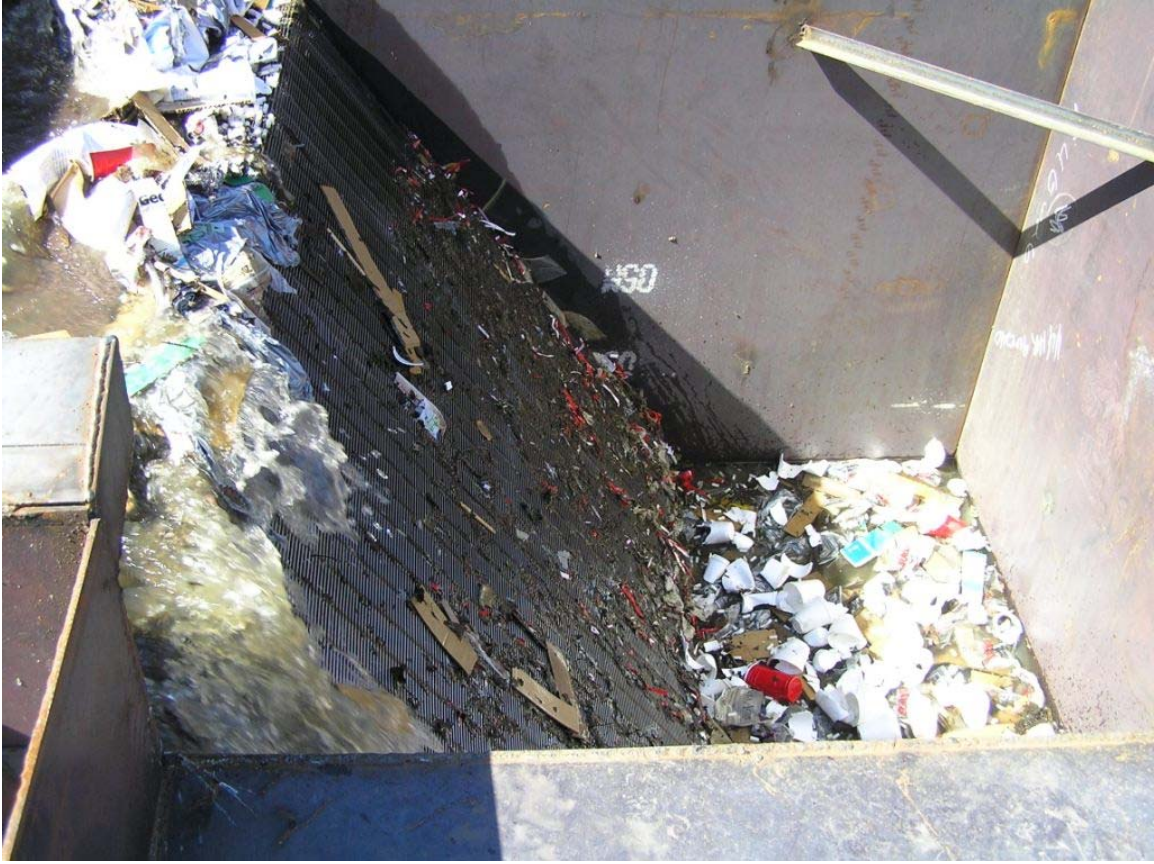
Fig. 6.38: Clogging of screens for Q=1.1 cfs and 50% loading.
