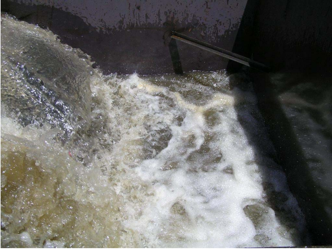
Fig. 6.26: Water level rise in gross solids storage tank for Q=7.06 cfs.
