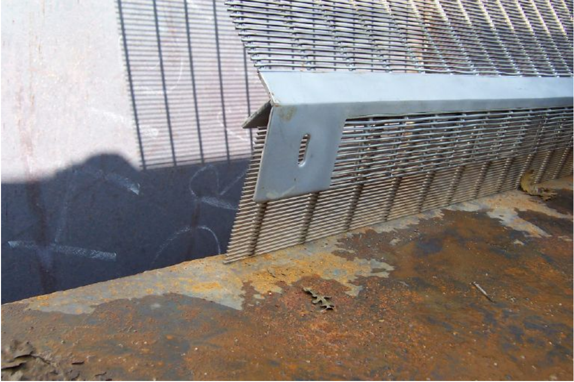
Fig. 5.3: Detail of the screen where it meets the sloped litter storage area.
