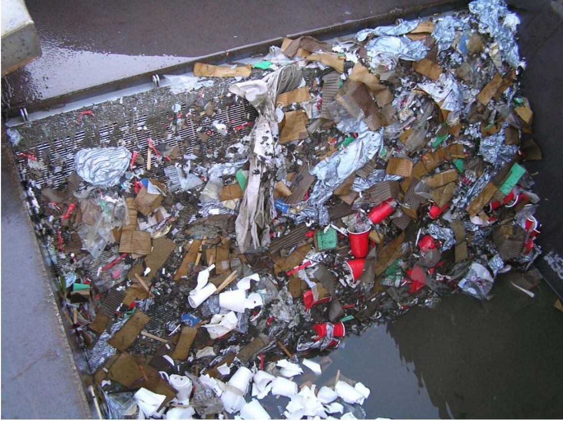
Fig. 6.50: Aftermath of Q=5.5 cfs and 50% loading.
