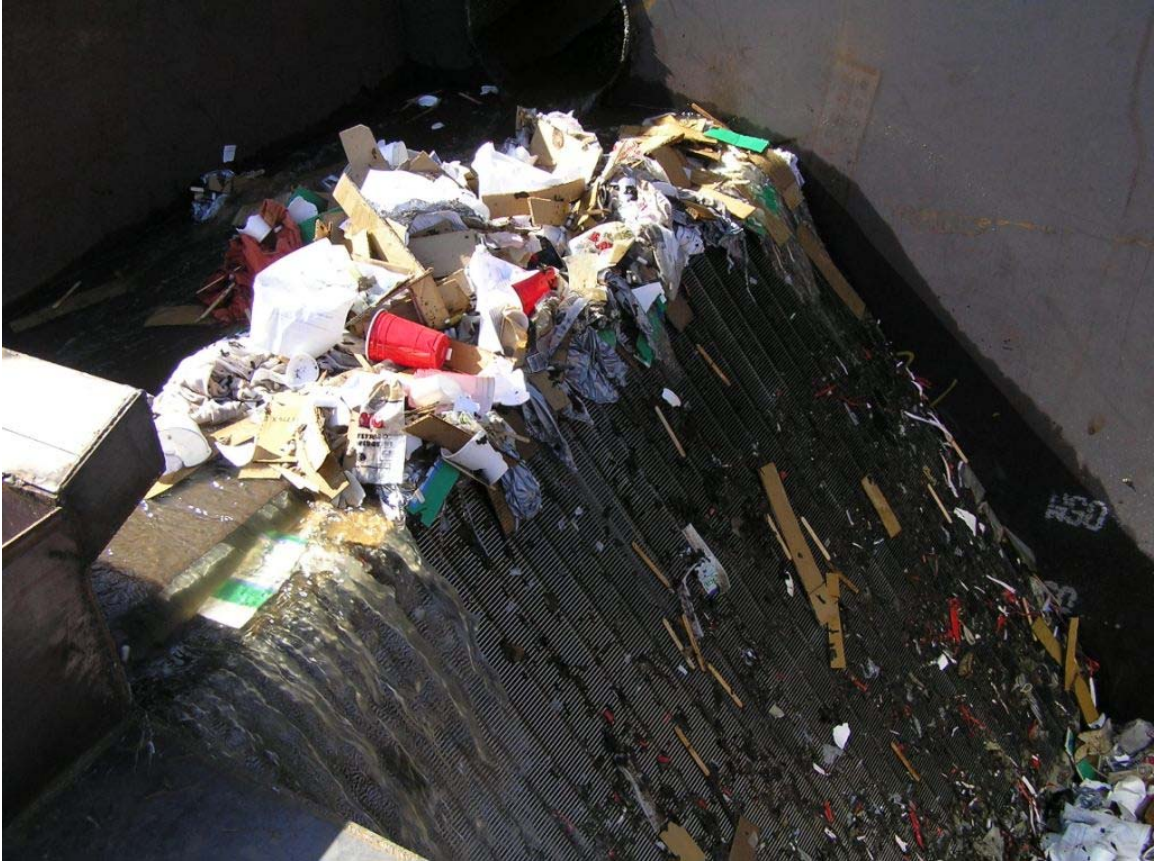
Fig. 6.42: A view of screen operation for Q=1.1 cfs and 90% loading.
