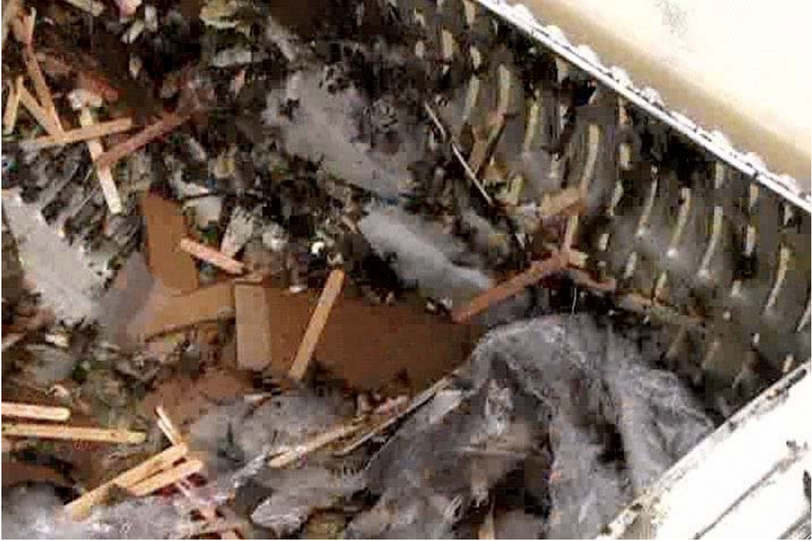
Fig. 4.60: loss of conveyance through louvers due to accumulation of gross solids.
