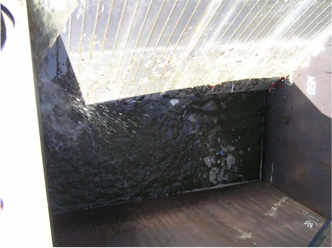
Fig. 6.9: Deflected flow into gross-solids storage area.
