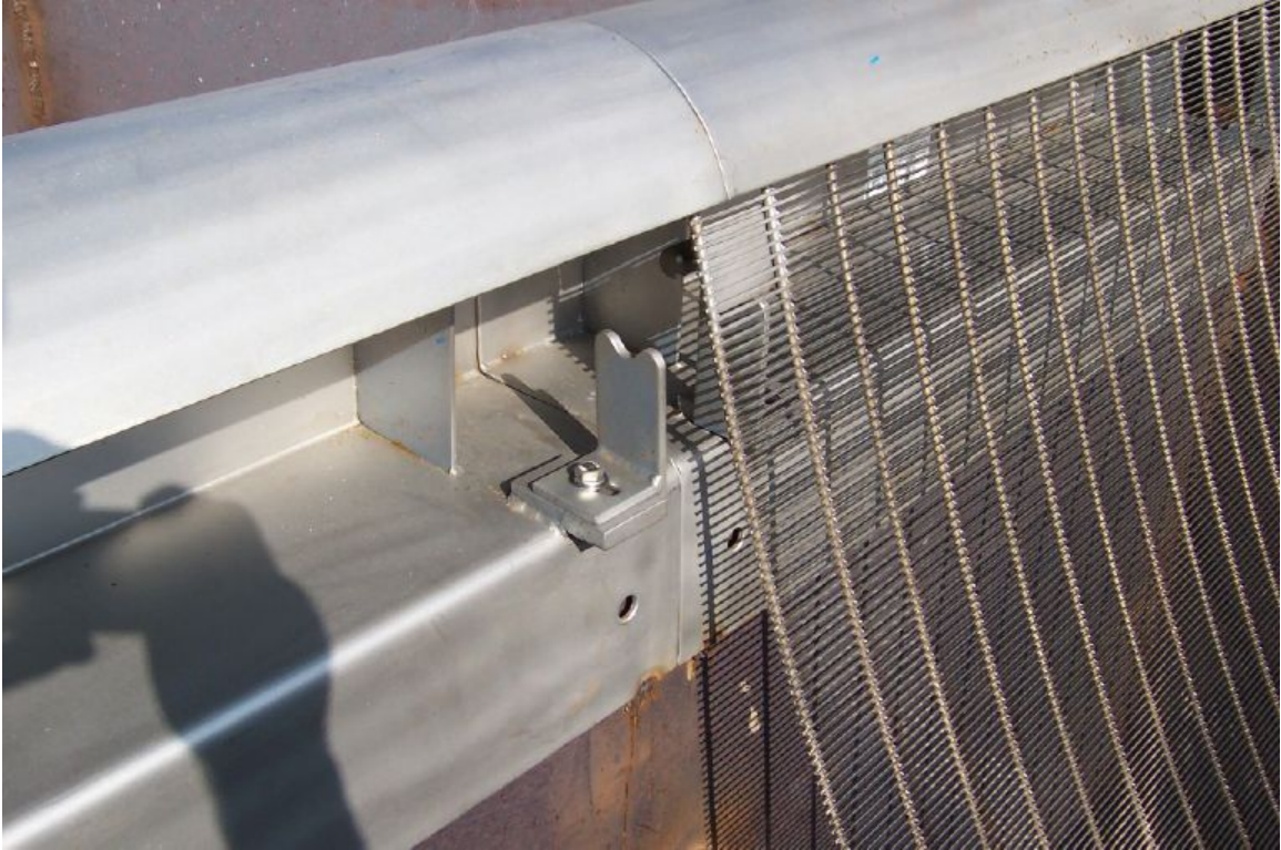
Fig. 5.2: A close-up of the parabolic screen attached to a weir.
