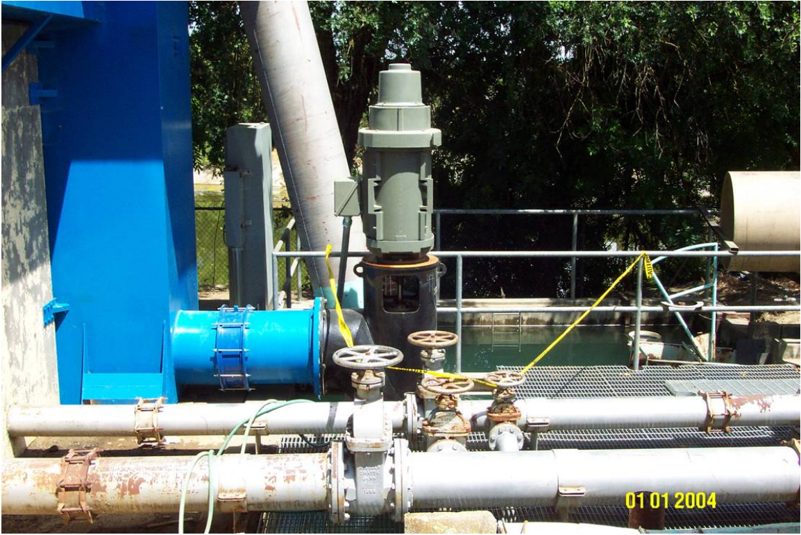
Fig. 2.3b: View of sump, pump, and pipes for return flow.
