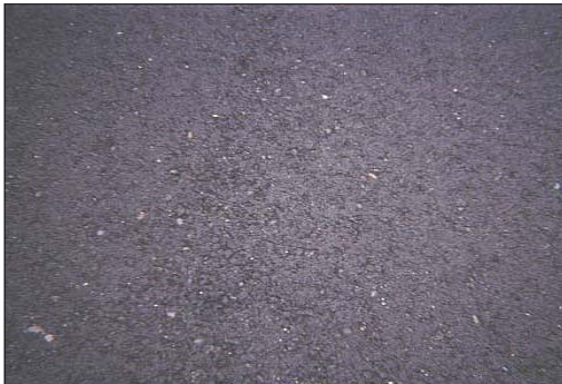
Figure 4: Unsuitable Surface, Dense Graded HMA With Closed Surface
