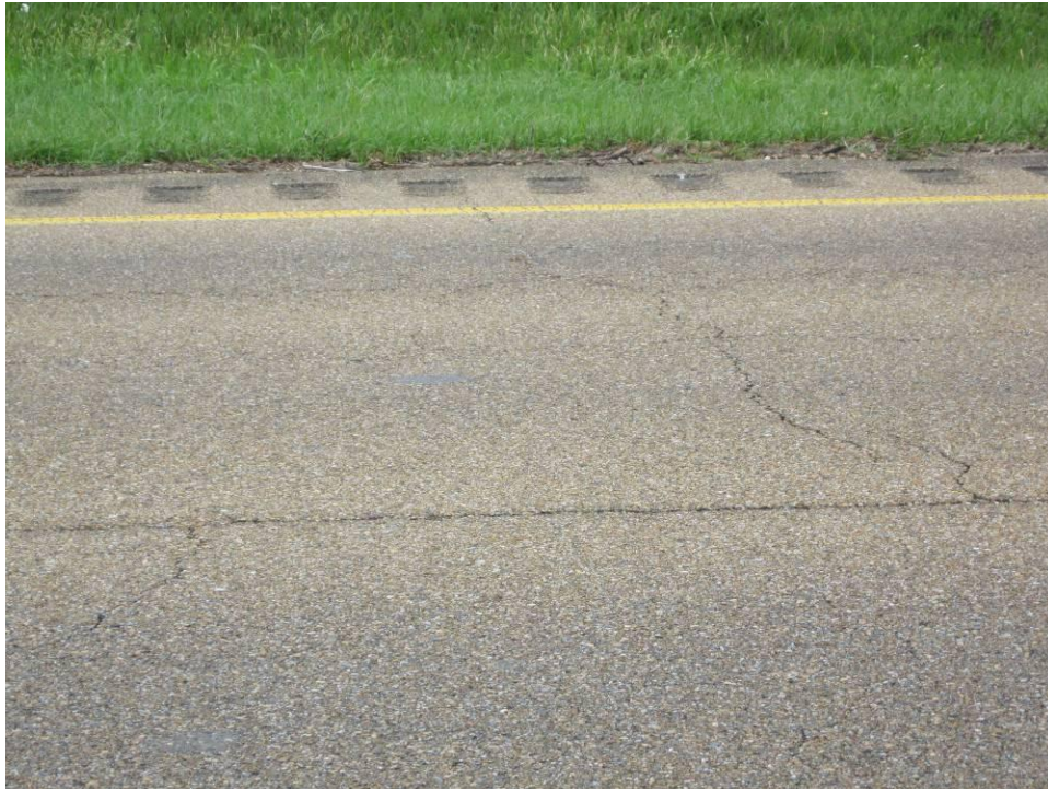
Figure 5: Premature Cracking Potentially Caused by Absorption Issues (South)
