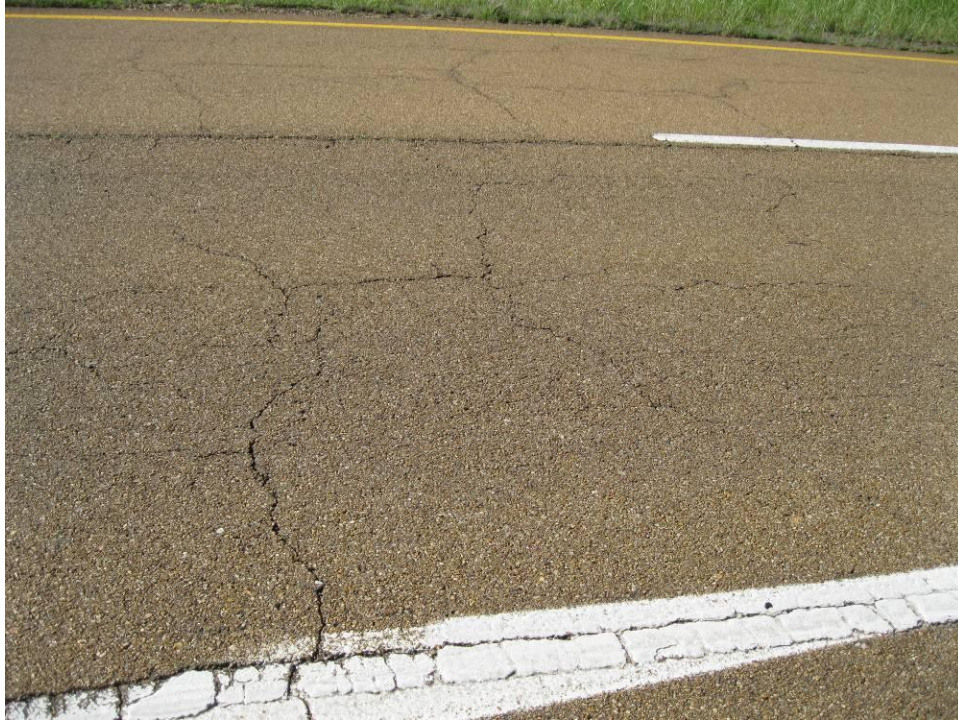
Figure 4: Premature Cracking Likely Caused by Absorption Issues (North)
