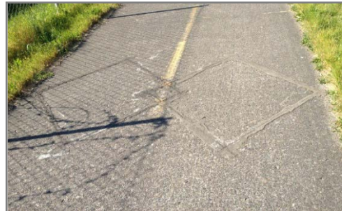
d. Double Diamond Bicycle Loop Detector on the I-205 Path at SE Yamhill St., Portland, OR
