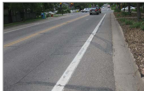
f. Parallelogram Loop Detector Used for Bike Lane Signal Actuation Loop in Boulder, CO
