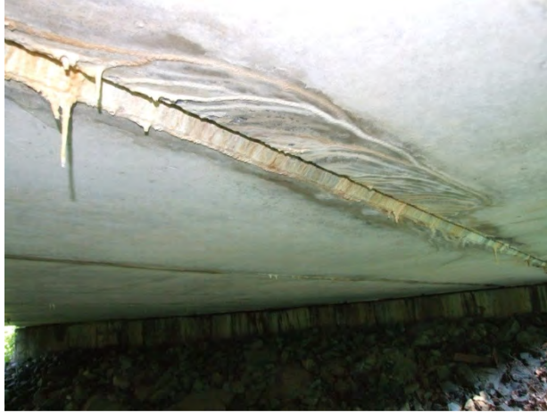
Figure 20. Result of Moisture Penetrating Between Two Box Beams
