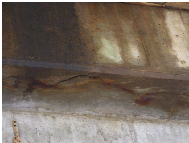
Figure 22. Evident Corrosion Along Bottom of Pier Cap Initiating Spalling of the Concrete
