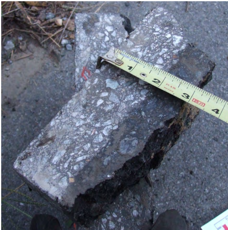
Figure 19. Asphalt at Location 4 Showing 1-in of Moisture Along Bottom, Which Was Adjacent to Overlay
