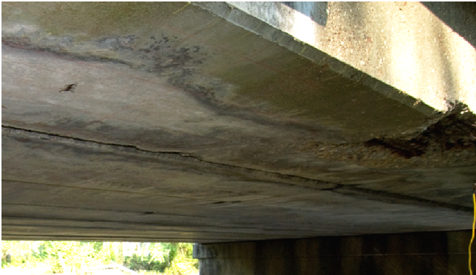
Figure 25. Bottom Side of Box Beams Showing Smooth Finish That Is Ideal for Use of Impact Echo Scanner
