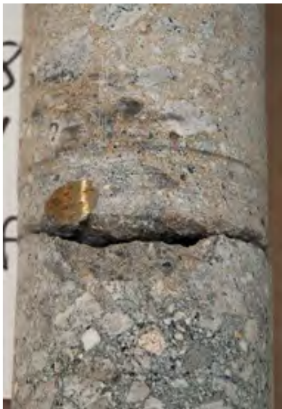
Figure 8. Actual Core Associated With Figure 7 Confirming Predicted Delamination
