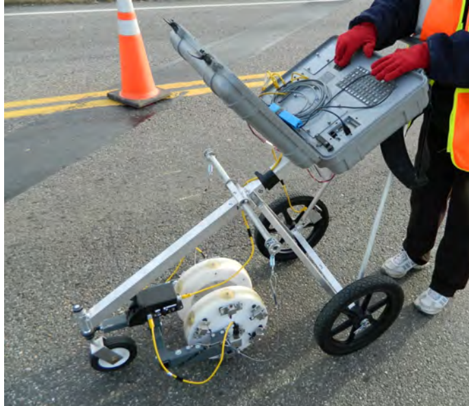
Figure 5. Photograph of Bridge Deck Scanner. Impactor solenoids on sides of wheels and brass displacement transducers spaced every 6 in aligned for impact echo test and spectral analysis of surface waves test.
