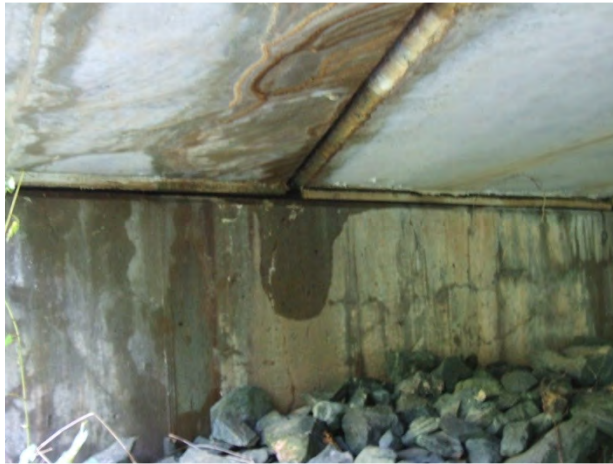
Figure 21. Evident Moisture Penetration on Abutment
