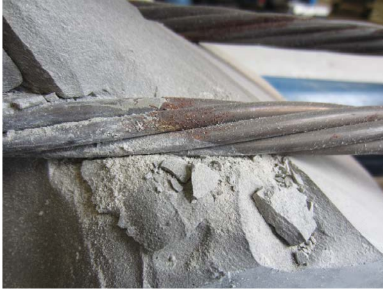
Figure 209. Photo. Exposed strand at the void/grout interface of 0.08 percent chloride multi-strand specimen.
