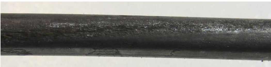
Figure 247. Photo. Crevice corrosion between two stressed wires on 0.4 percent chloride concentration multi-strand specimen (mean pit depth = 4.5 mil and maximum pit depth = 8.0 mil).
