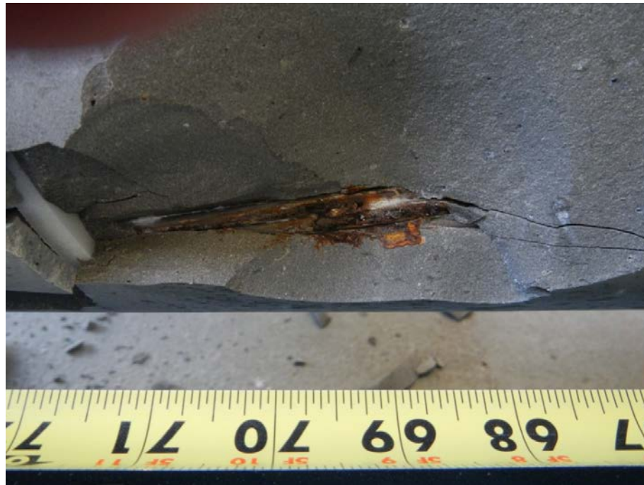
Figure 229. Photo. Active corrosion of a stressed strand inside the 2.0 percent chloride grout 70 inches from the lower anchorage.
