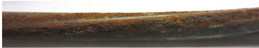
Figure 63. Photo. Example of heavy rust on the extracted wires.
