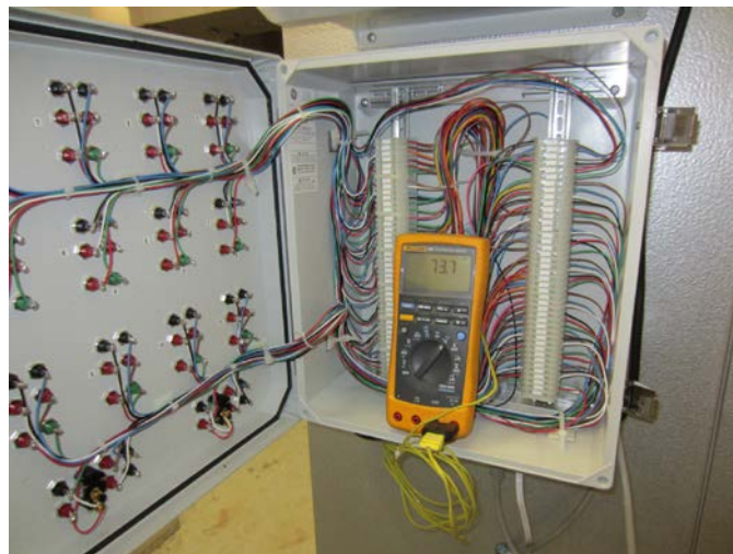
Figure 6. Photo. Data collection terminal cabinet.
