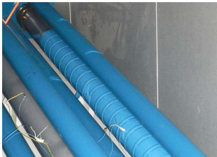
Figure 51. Photo. Cracked duct of 0.8 percent chloride multi-strand specimen after repair.
