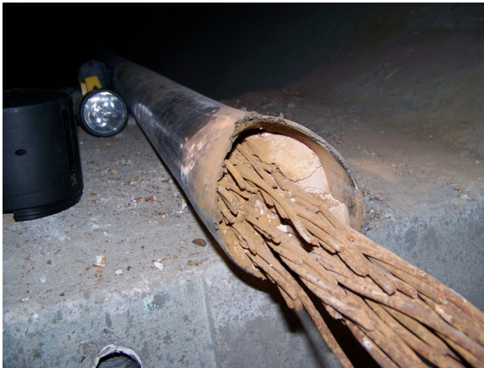
Figure 264. Photo. Failed external PT tendon of Verina-Enon bridge in Virginia.
