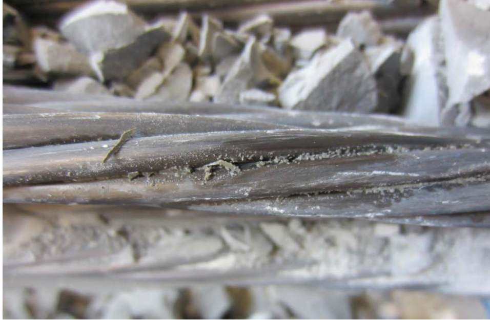
Figure 233. Photo. Wet and soft grout found in 0.8 percent chloride multi-strand specimen.
