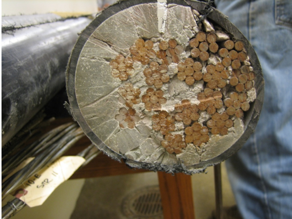
Figure 265. Photo. Other matching end of the retrieved tendon sample shown in figure 264.
