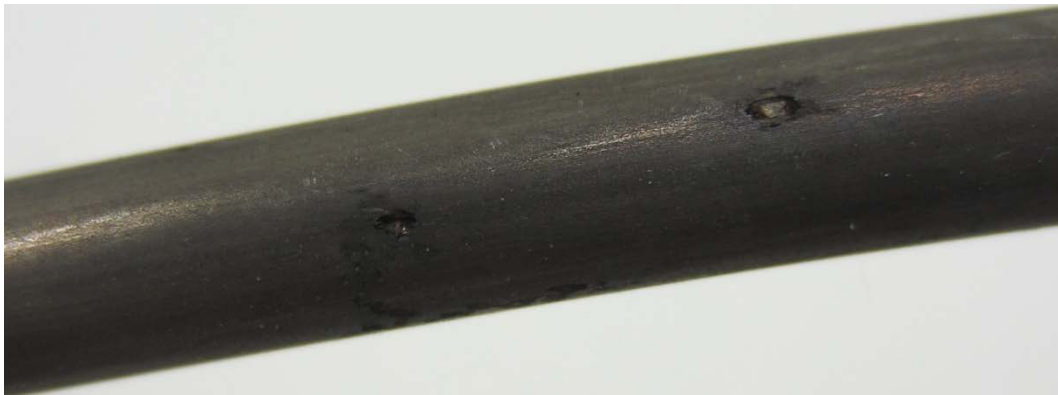
Figure 239. Photo. Stressed and fully grouted 0.8 percent chloride single-strand specimen (pit depth = 4.7 mil).
