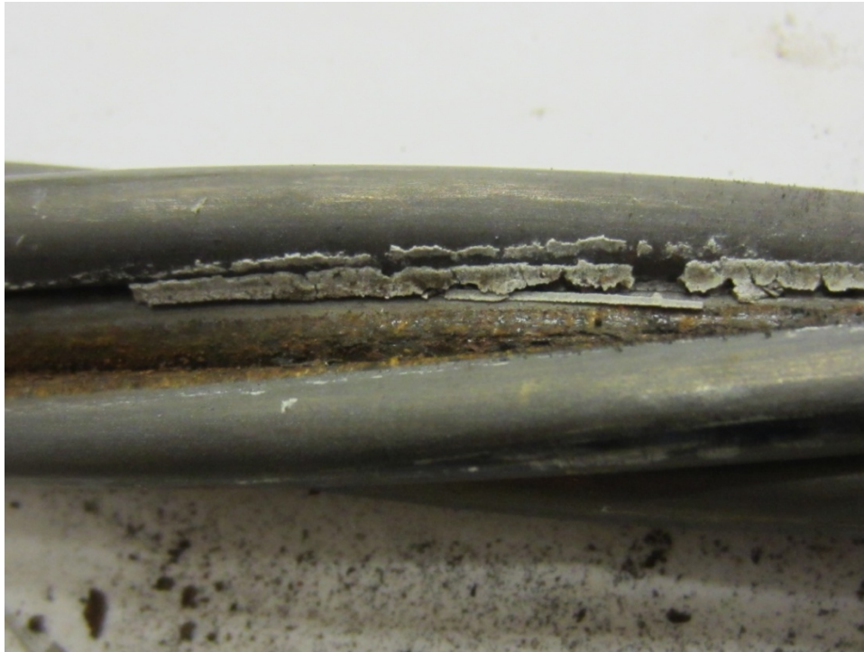
Figure 235. Photo. Grout fragment found inside an interstice surrounded by corroding wires.
