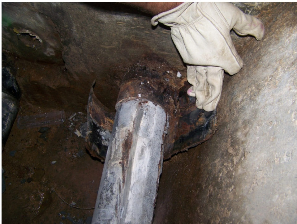
Figure 266. Photo. Corroding PT tendon of Verina-Enon bridge in Virginia.
