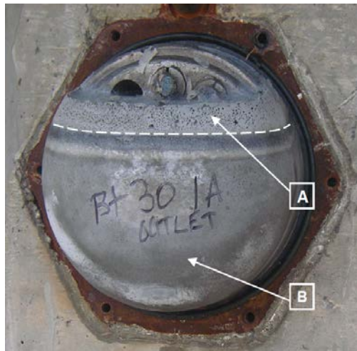
Figure 2. Photo. Chloride-contaminated grout in the straddle caps for Carbon Plant Road bridge. (5)
