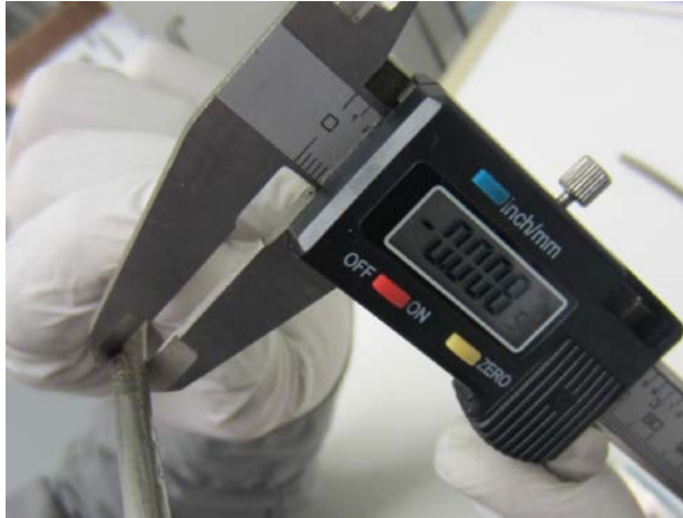
Figure 78. Photo. Section loss measurement in a severely corroded area.
