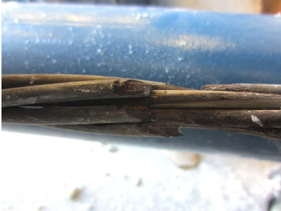
Figure 220. Photo. Close-up view of the severely corroded strand shown in figure 219.
