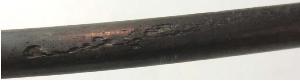
Figure 248. Photo. Crevice corrosion between two stressed wires on 0.8 percent chloride concentration multi-strand specimen (mean pit depth = 4.5 mil and maximum pit depth = 6.0 mil).
