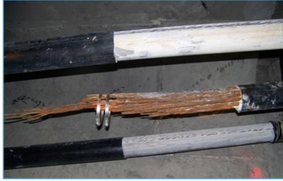
Figure 18. Photo. Example of PT tendon failure due to macro-cell corrosion—Verina-Enon bridge in Virginia after 17 years in service.
