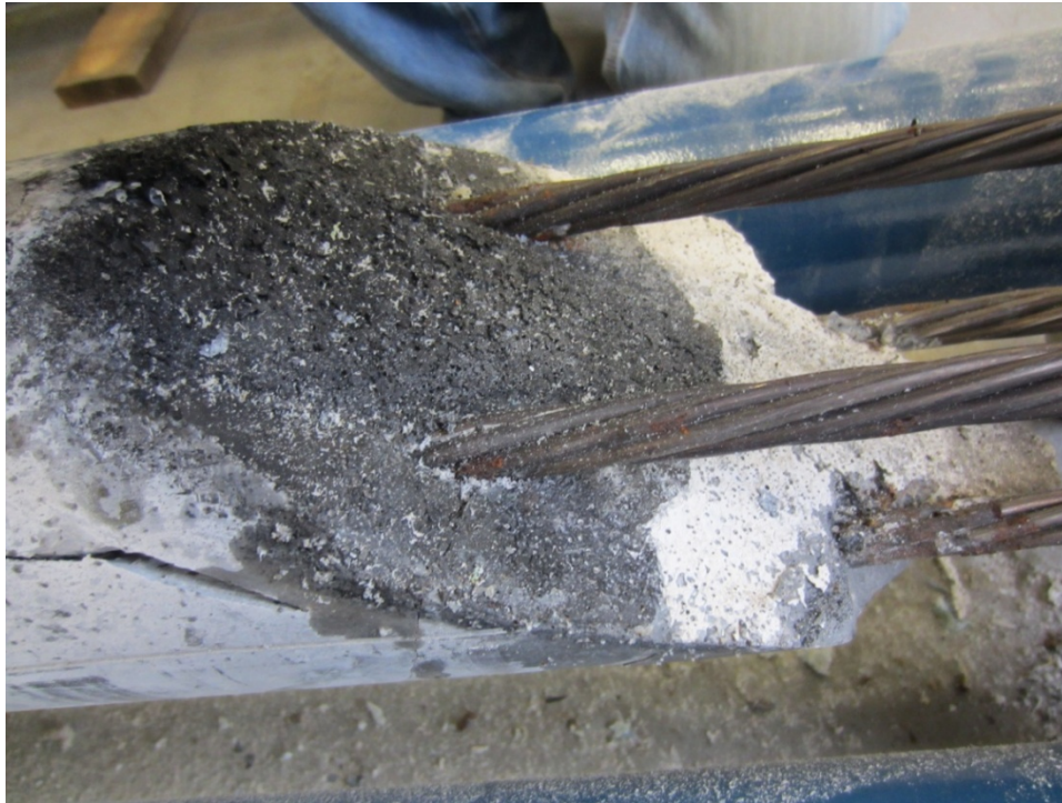
Figure 213. Photo. Strands at the void/grout interface of 0 percent chloride multi-strand specimen.
