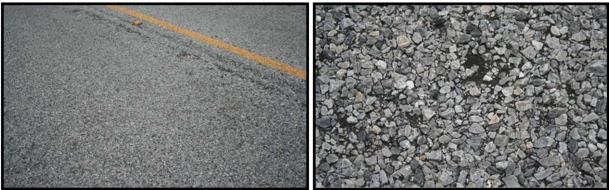
Figure 5.13. Hwy 44 Section 1 Two Year Survey (09/18/2013)
