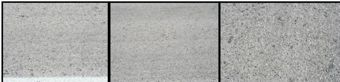
Figure 5.21. Hwy 366 Section 2 Two Year Survey (09/19/2012)
