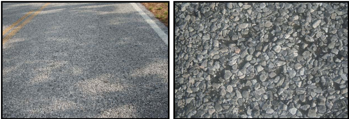
Figure 5.14. Hwy 44 Section 2 Two Year Survey (09/18/2013)
