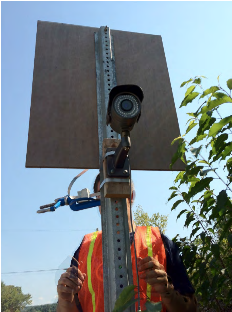
Figure 5 Video Camera Installation near Richmond iCone 2, in the Eastbound 25-mph Section
