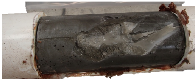
Figure 117—Soft grout located in segregation canal
