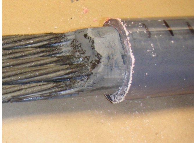
Figure 60—Soft grout found at top of tube containing PT4-1 in which the grout hose was filled with 2 gallons of water prior to injection
