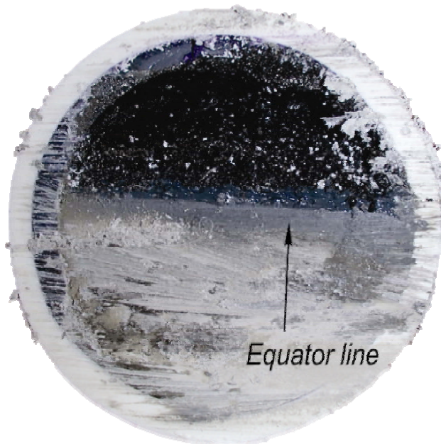
Figure 119—Equator line separating hard cement from soft grout (PT grout)
