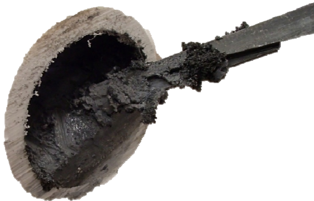
Figure 109—PT4-6 soft grout
