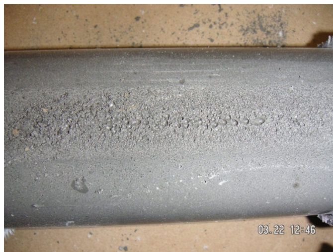
Figure 50—Porous surface observed in top half of tube containing PT1-2 at MWD
