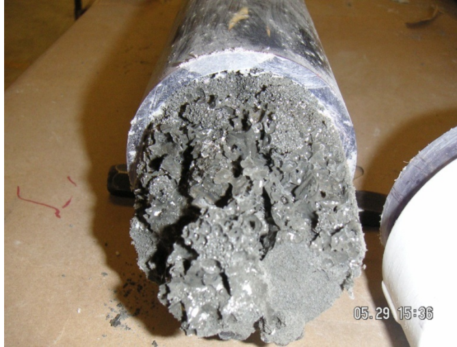
Figure 51—Porous grout observed in PT1-2 at 1.15·MWD
