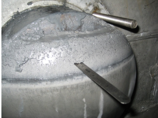
Figure 2—Soft grout sample identified in field by FDOT
