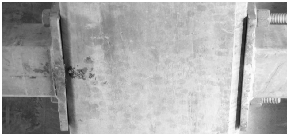
Figure 3.5 Damage to End Plates of Steel Diaphragm Members
