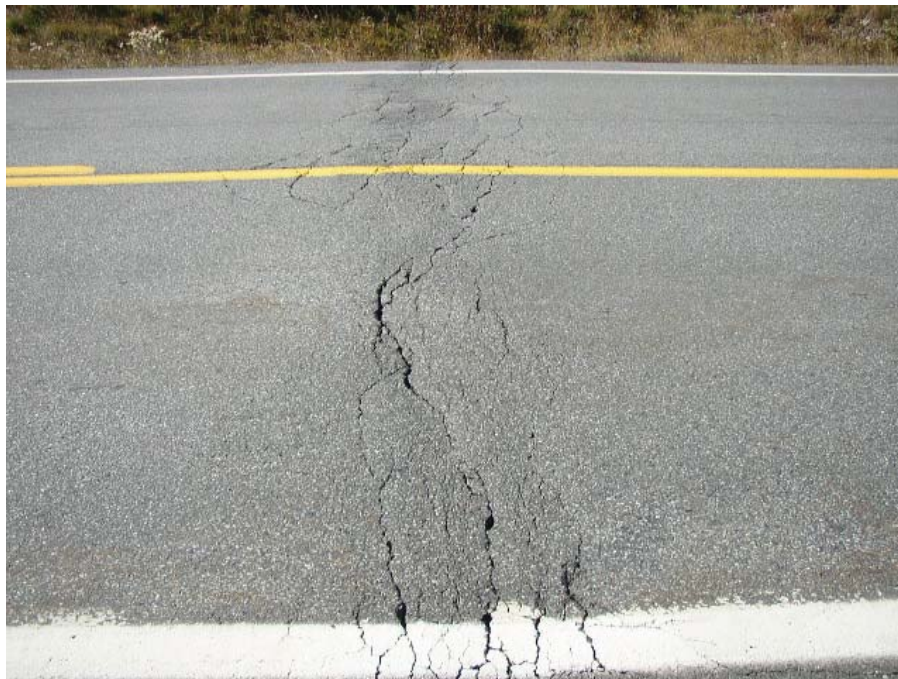
Photo 5: Cross Pipe 4 Transverse Cracking
