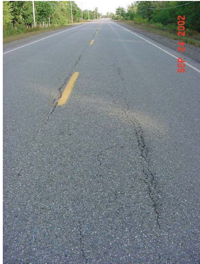
Photo 2. Experimental 1 Centerline & Load Cracking
