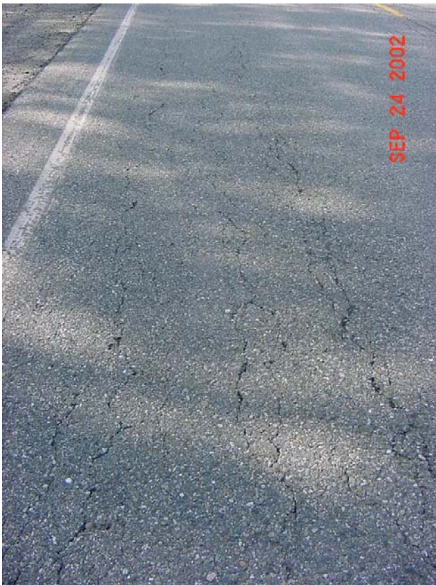
Photo 3. Control 2 Moderate Load Cracking
