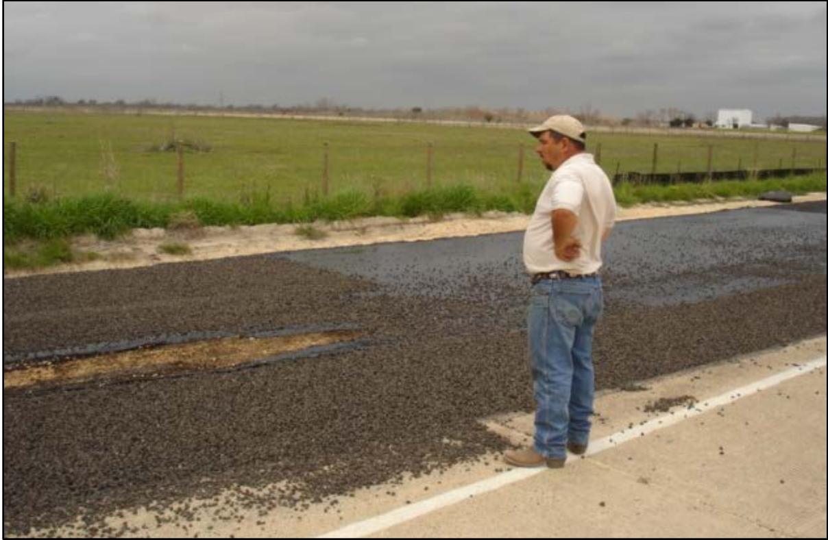
Figure 48. Strip of Grade 3 Course that Peeled Off at South Access Ramp.
