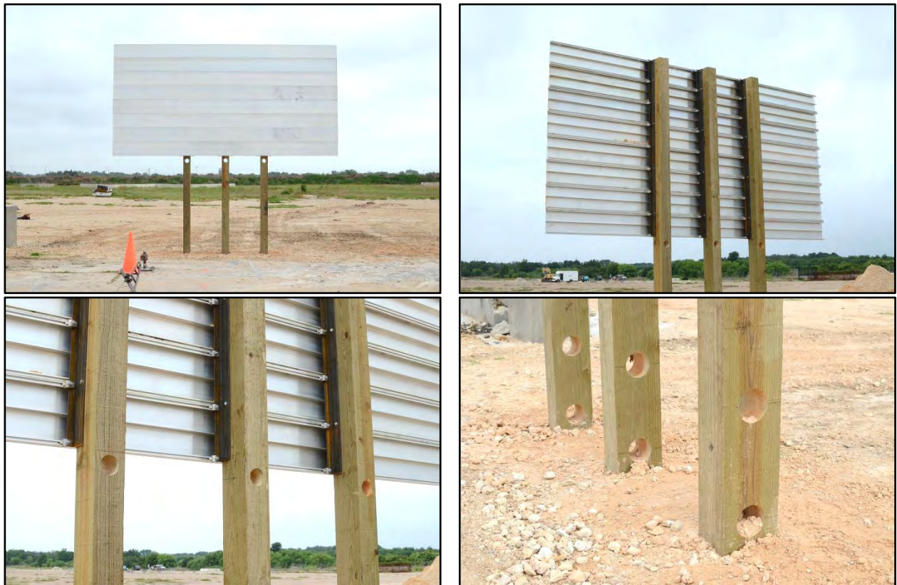
Figure 4.2. Direct Embedded Wood Support Temporary Guide Sign System before Test Nos. 467823-1 and 467823-2.
