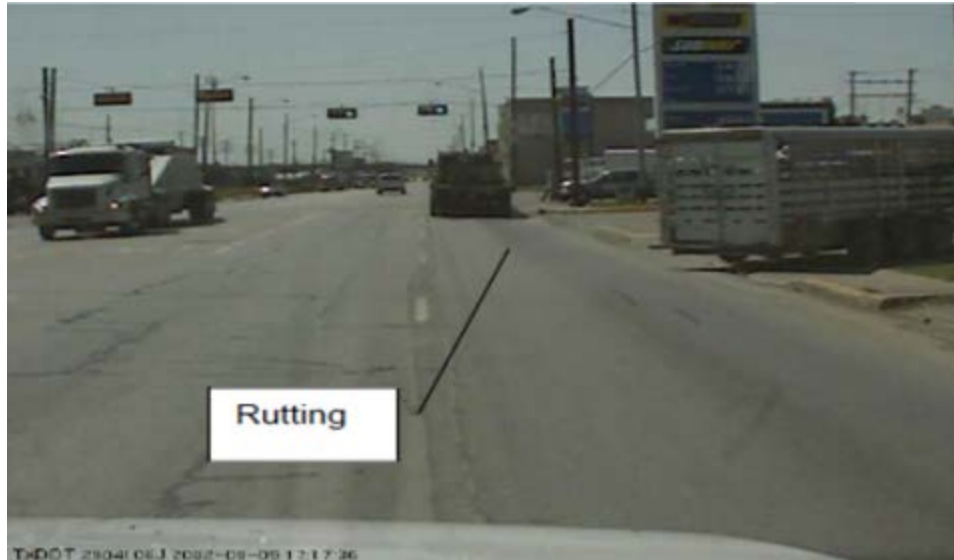
Figure 1-3. Surfacing Rutting on Anderson Street in Bryan District (over 0.5 inches Surface Rutting).
