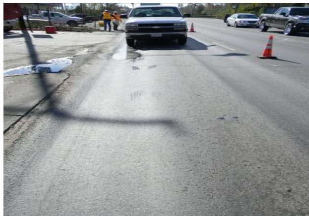
Figure 1-2. Severe Surface Rutting on US 96 in Beaumont District (over 1.5 inches Rut Depth).
