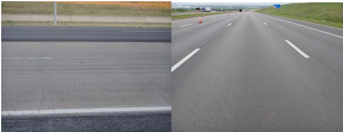
(a) Fine Cracks on CRCP
