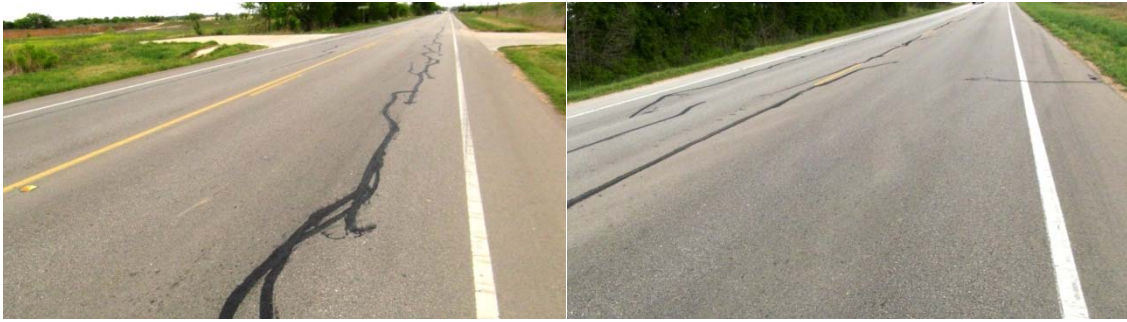
Figure 3. Observed Cracks on Sections 5 and 6.
