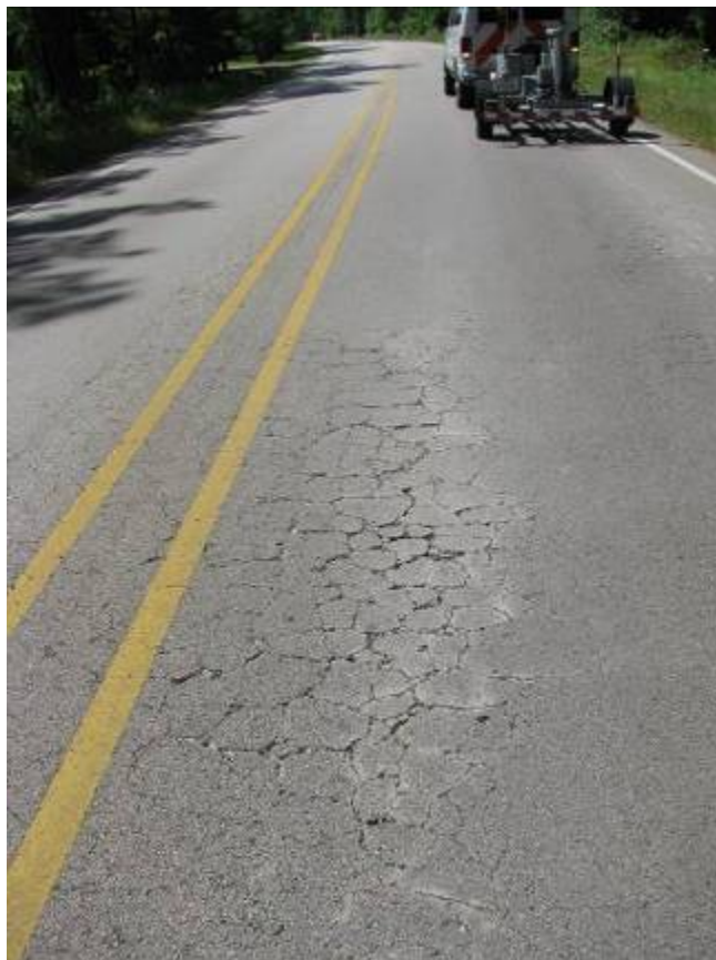
Figure 8. Alligator Cracking at South End of Project.
