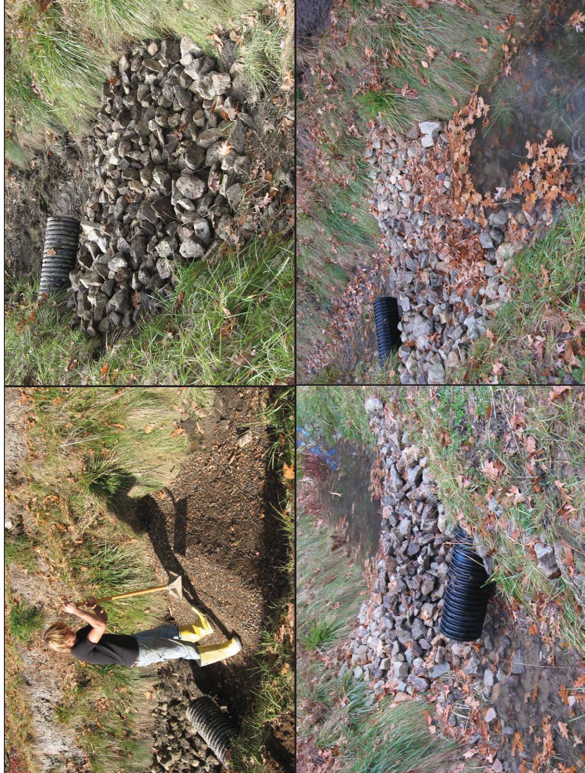
Figure 5: Filter Berm Installation at UNHSC (Top left to right clockwise; Filter core placement; Looking downstream after installation; Looking downstream during rain event; (Culvert is not part of berm structure and is located downstream of installation)
