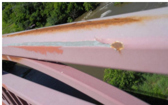
Baraboo bridge railing damage due to freezing
