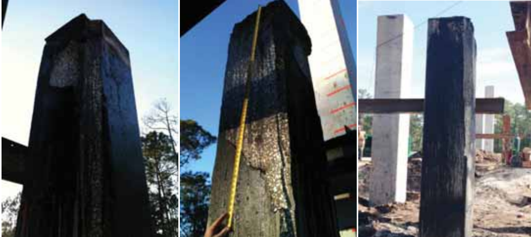
Figure 12 – Diesel Covered Pile with Spalled Sections
