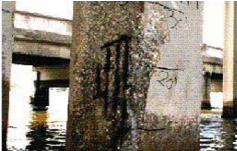
Figure 1.1: Splash zone corrosion
