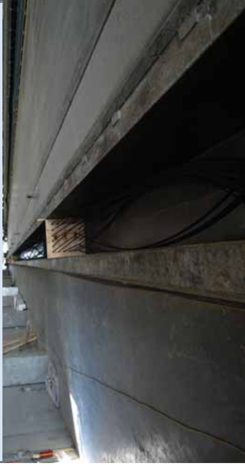
Strands in position. Note the adjacent, previously-cast pile in the self-stressing forms.
