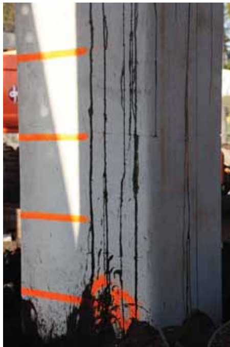
Figure H.38: Horizontal (tension) crack in Pile 2
