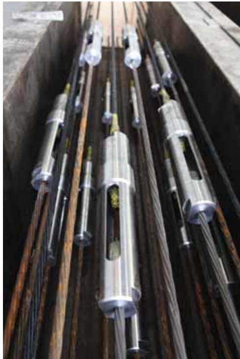
Figure H.25: Showing staggered couplers and close-up of coupler, with CFCC strands already stressed
