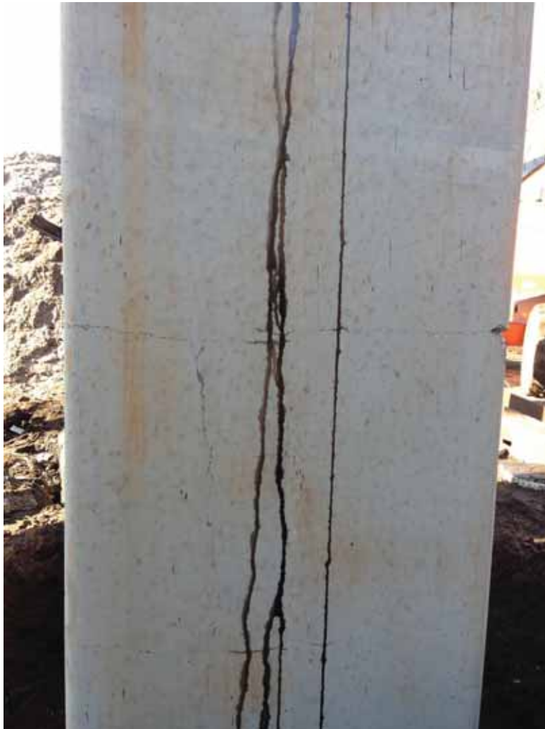
Figure H.39: Horizontal (tension) crack in Pile 2, on other side
