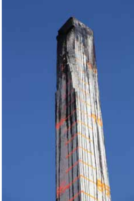
Figure H.37: Concrete spalling on head of Pile 2 during driving
