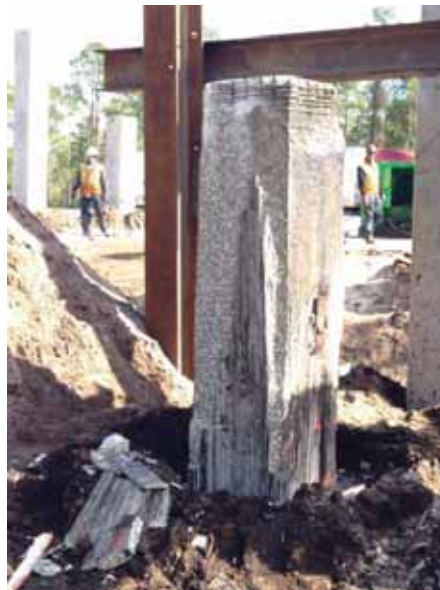
Figure 14 – Spalling near the Top of Pile N2
