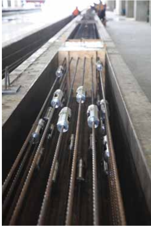
Figure H.24: Showing staggered couplers, with CFCC strands already stressed, looking from stressing end
