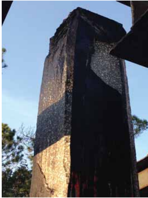
Figure H.35: Leaked diesel and concrete spalling on head of Pile 1 after being driven
