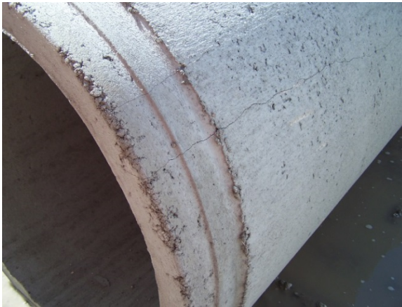
Figure 3-11: Hairline Crack on RCP
