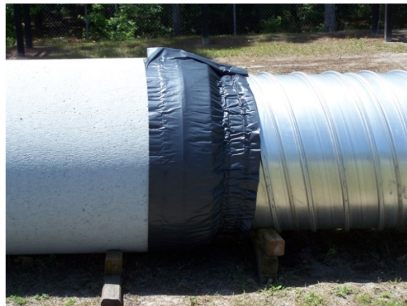
Figure 3-16: Dissimilar Pipe Coupler at RCP-to-CMP Junction
