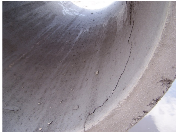
Figure 3-12: Larger Crack on RCP
