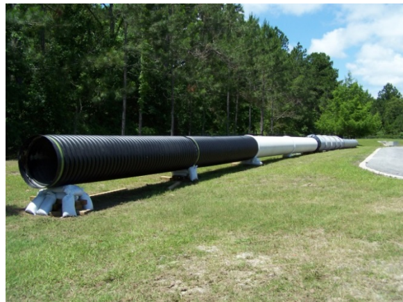
Figure 3-14: Elevated Pipe Course Run
