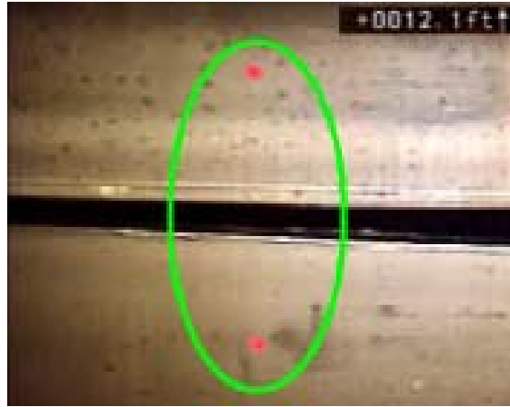
Figure 2-8: Measurement of a Joint Gap with a Video-Micrometer – Using Two Laser Beams (from C-Tec Presentation)
