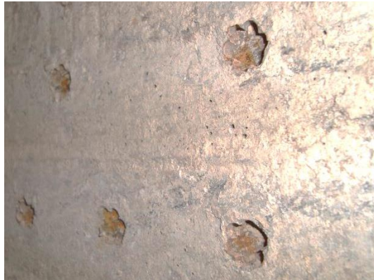
Fig. 4.17 Prestressing steel pulled into the girder at failure
