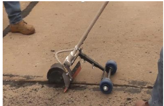
Figure 3.4 Removing old sealant from a concrete joint with a router bit attachment
