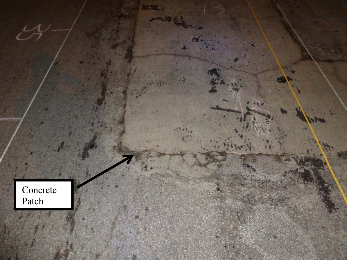
Figure 3-1 Bridge A0569 Concrete Patch and Deteriorated Asphalt Overlay Observed During Field Investigation
