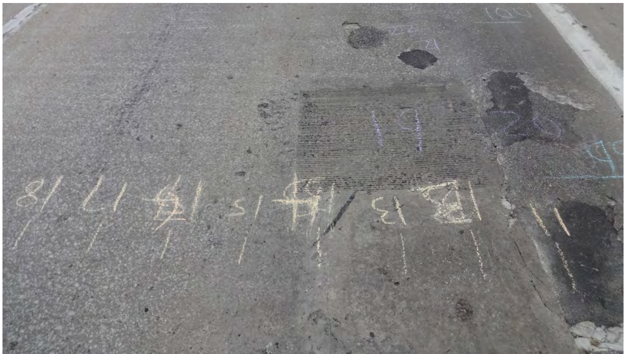
Figure 3-7 Bridge A2111 Typical Deck Condition Observed During Field Investigation
