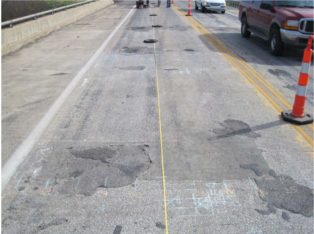
Figure 3-5 Bridge A1297 Typical Deck Condition Observed During Field Investigation
