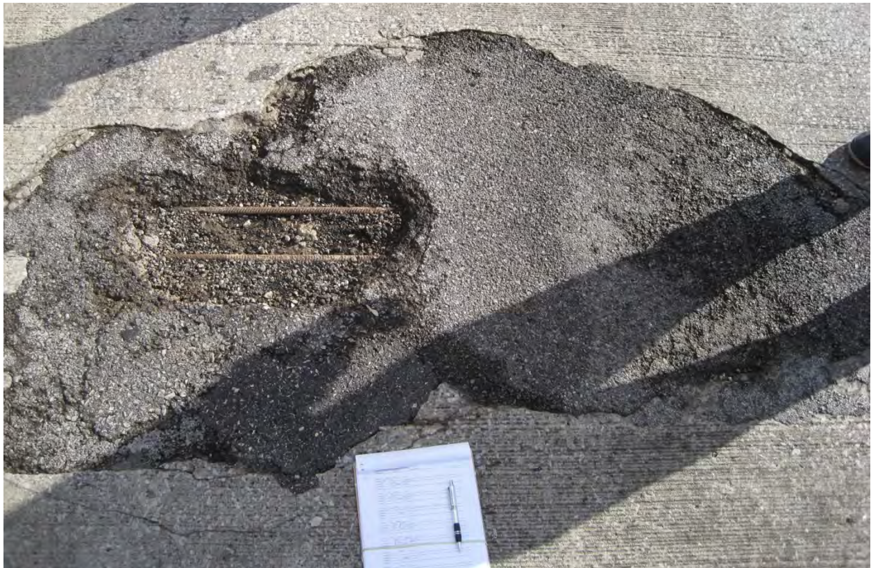
Figure 3-4 Bridge A1193 Typical Asphalt Filled Pothole Observed During Field Investigation
