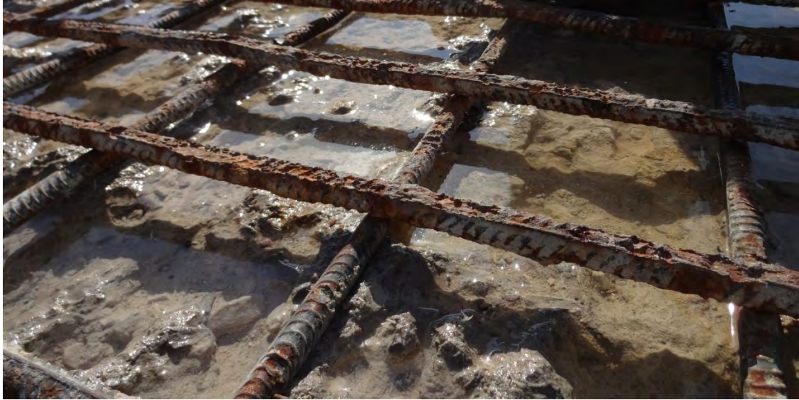
Figure 6-2 Corroded Rebar Exposed After Removal of Loose and Deteriorated Concrete by Hydro Demolition
