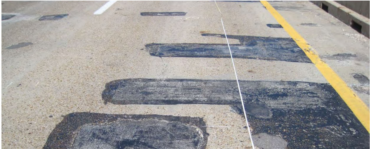
Figure 3-6 Bridge A1479 Typical Deck Condition Observed During Field Investigation
