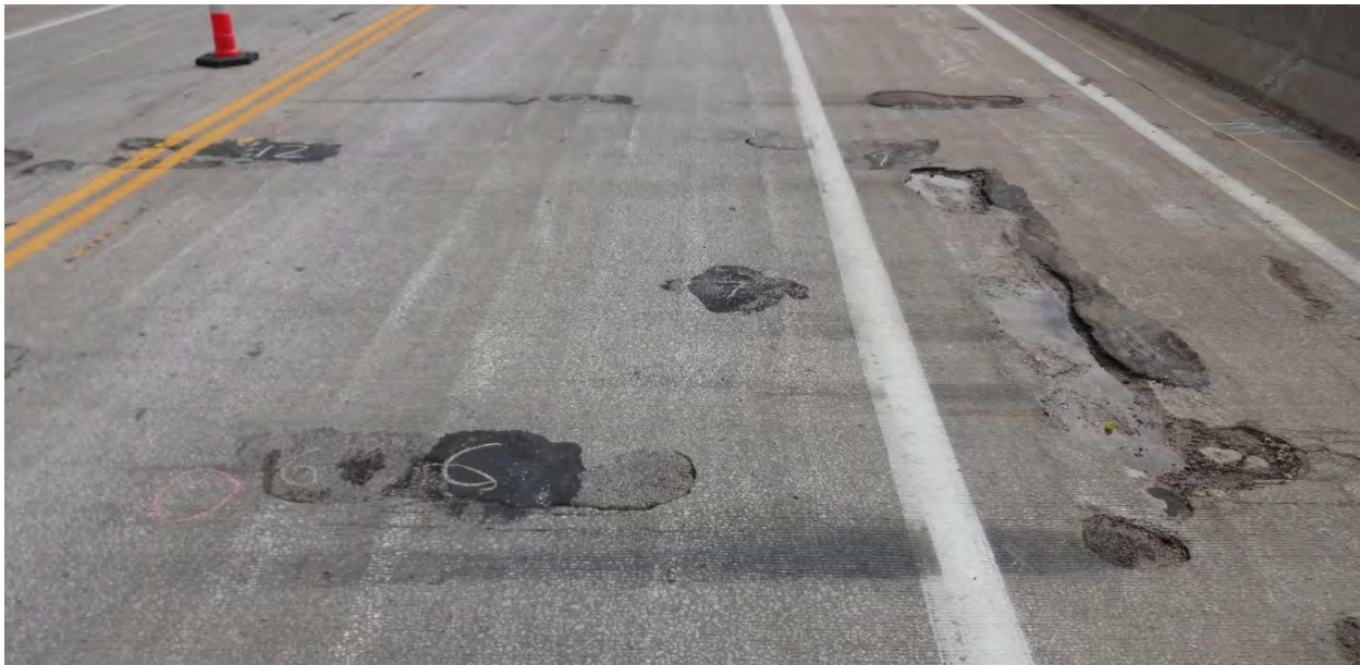
Figure 3-9 Bridge A3017 Typical Deck Deterioration Observed During Field Investigation
