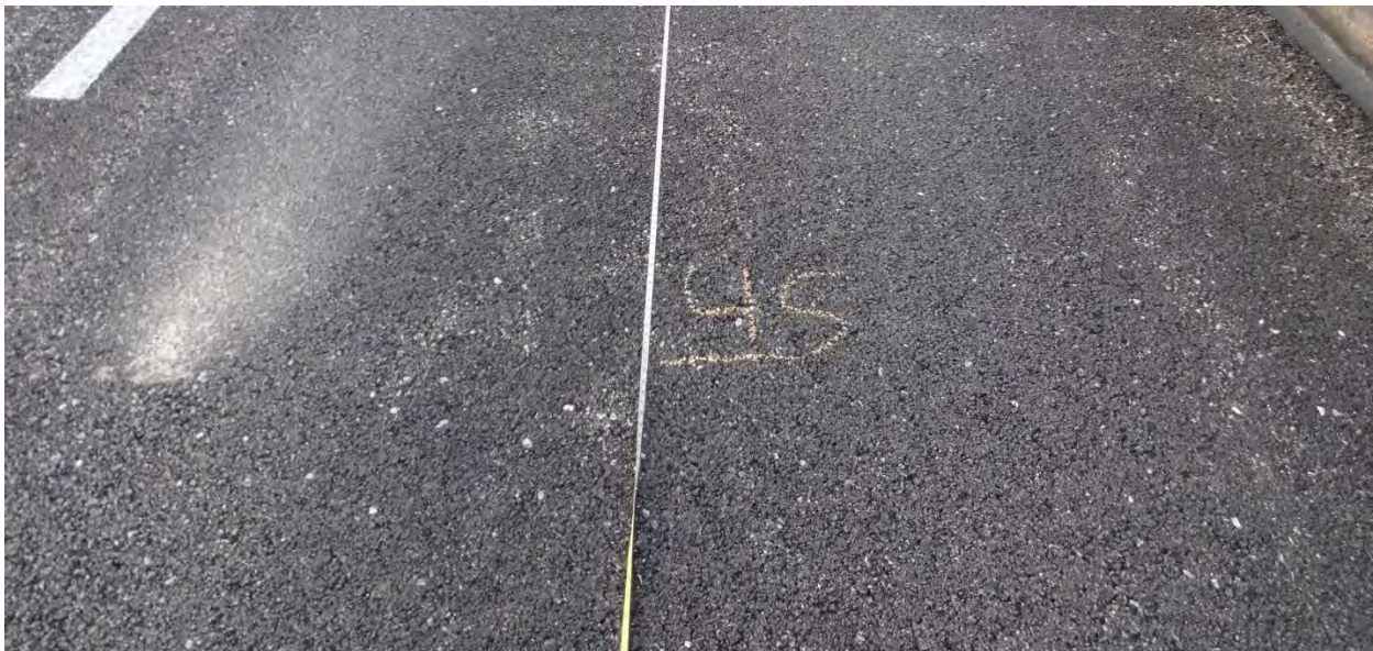
Figure 3-3 Bridge A1187 Deck Surface Observed During Second Investigation
